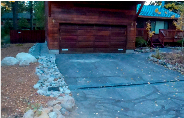
Trench drain placed at the foot of a driveway that slopes toward the street. The stormwater is moved into rock area at left where it can infiltrate. Image courtesy of Basile Management Practices.
