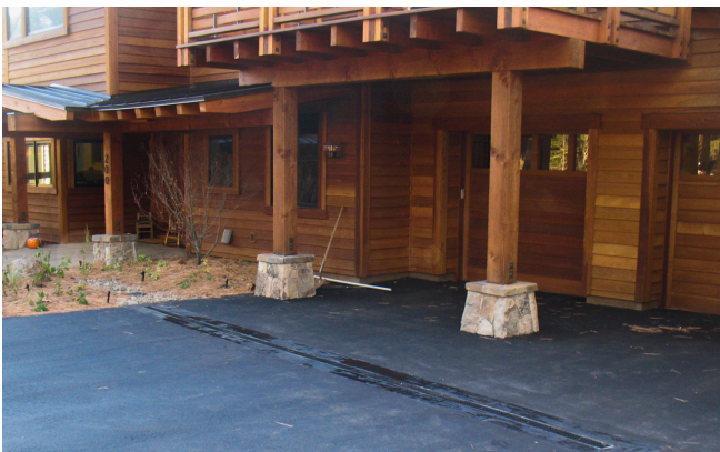
Trench drain placed at the foot of a driveway that slopes toward the home. The drain moves stormwater into garden at left. Image courtesy of Basile Management Practices, bmptahoe.com .
