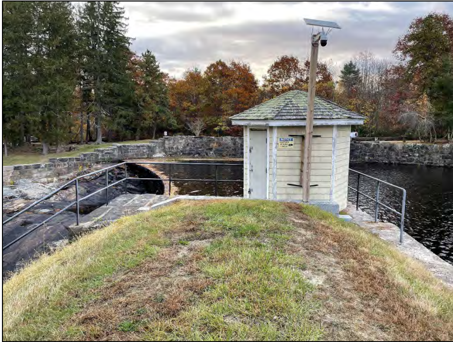
Photo No. 15.: Overview of the exterior of the gatehouse of the "Draw-Off" outlet system.
