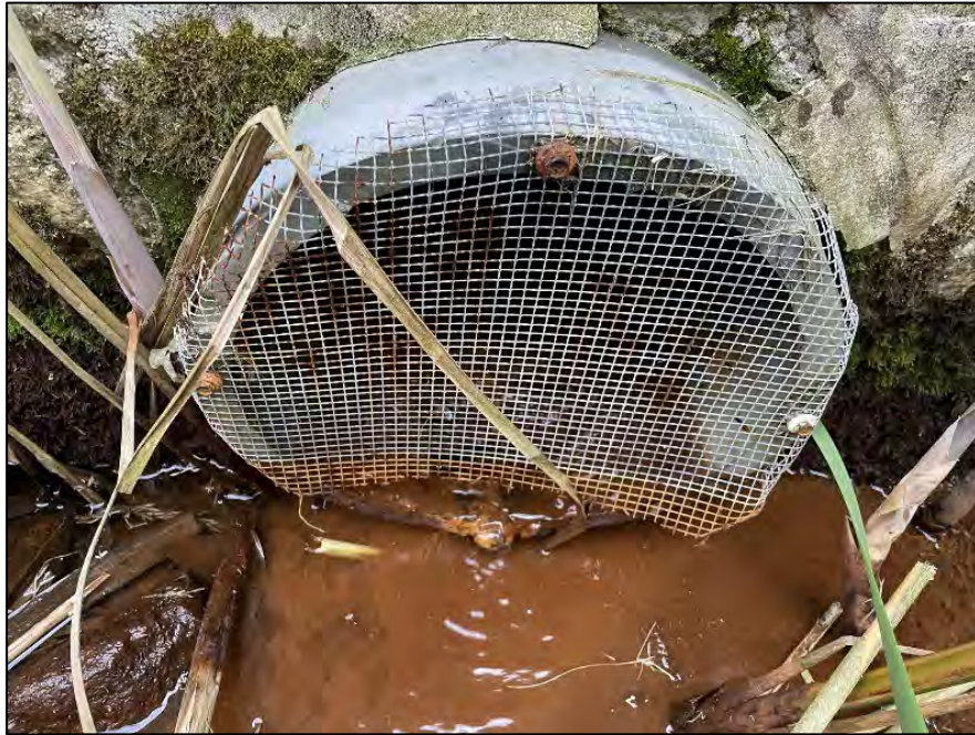
Photo No. 25.: Toe drain outfall at the "Mill Supply" low level outlet headwall. Note the iron oxide staining and the chewed-out bottom of the rodent screen.
