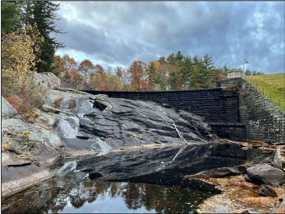
Photo No. 10.: Overview of the spillway from the downstream channel looking upstream.
