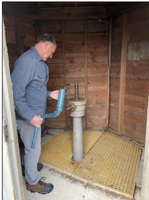
Photo No. 16.: Overview of the interior of the gatehouse of the "Draw-Off" outlet system..
