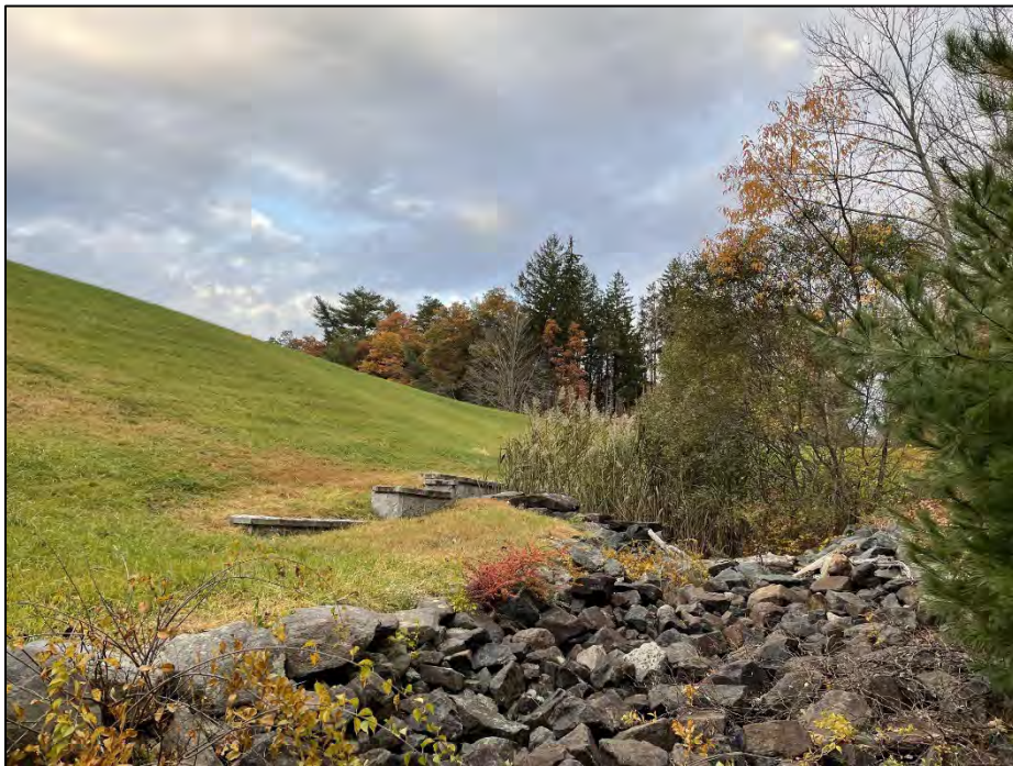
Photo No. 24.: "Old Mill Channel" riprap diversion swale that extends from the downstream channel to the "Mill Supply" outlet system to the downstream channel of the spillway.
