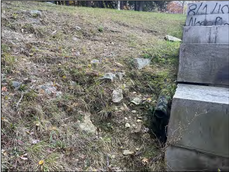
Photo No. 14.: Area of previously reported erosion at the end of the right downstream training wall of the spillway.
