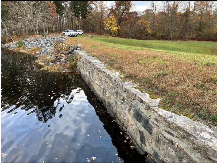
Photo No. 3.: Overview of the upstream side from the "Mill Supply" gatehouse looking left.
