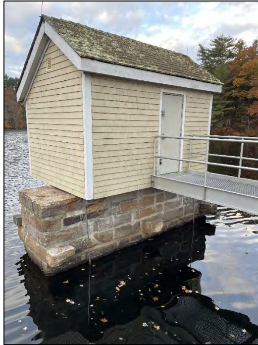
Photo No. 19.: Overview of the exterior of the gatehouse of the "Mill Supply" outlet system.
