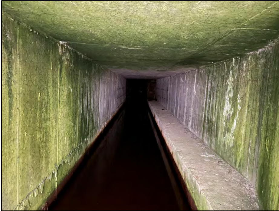
Photo No. 21.: View of the interior of the left discharge conduit of the "Mill Supply" outlet system from the downstream end looking upstream.
