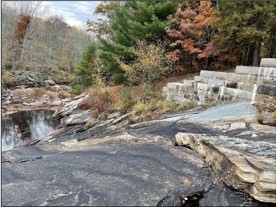
Photo No. 13.: Overview of the right downstream training wall of the spillway.
