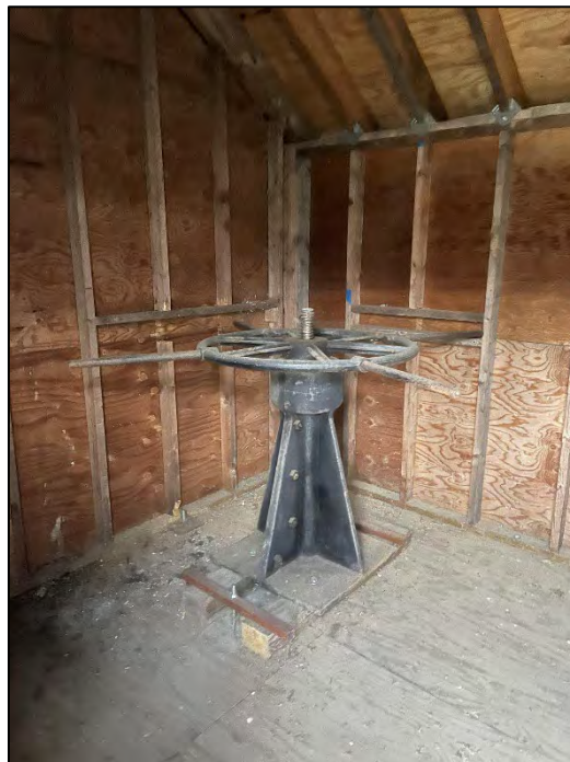
Photo No. 20.: Overview of the interior of the gatehouse of the "Mill Supply" outlet system.
