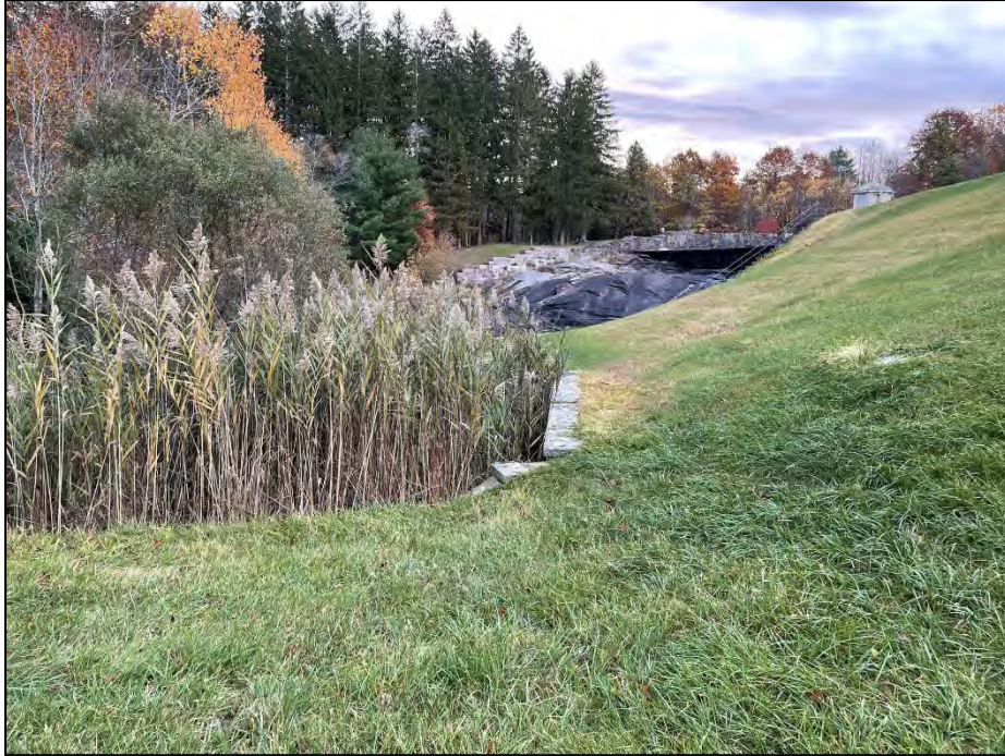
Photo No. 23.: Downstream headwall and channel of the discharge conduits of the "Mill Supply" outlet system.
