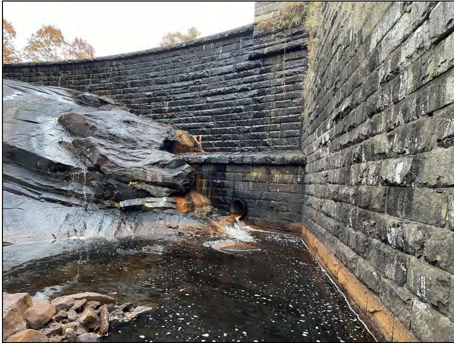
Photo No. 17.: View of the outlet end of the conduit of the "Draw-Off" outlet system.
