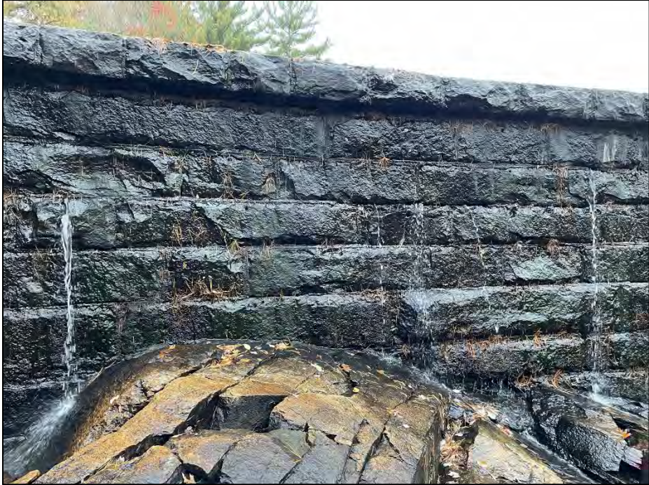
Photo No. 11.: Minor leakage through stone masonry blocks of the spillway.
