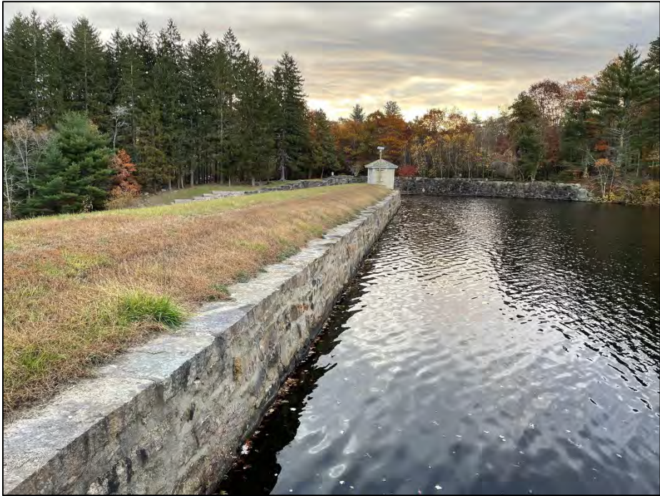
Photo No. 4.: Overview of the upstream side from the "Mill Supply" gatehouse looking right.
