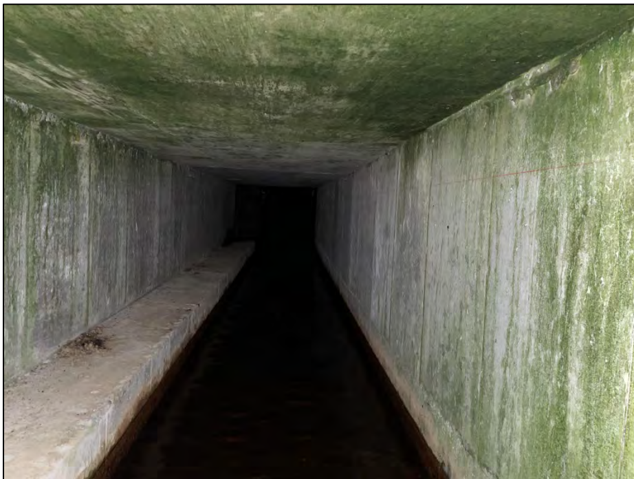
Photo No. 22.: View of the interior of the right discharge conduit of the "Mill Supply" outlet system from the downstream end looking upstream.
