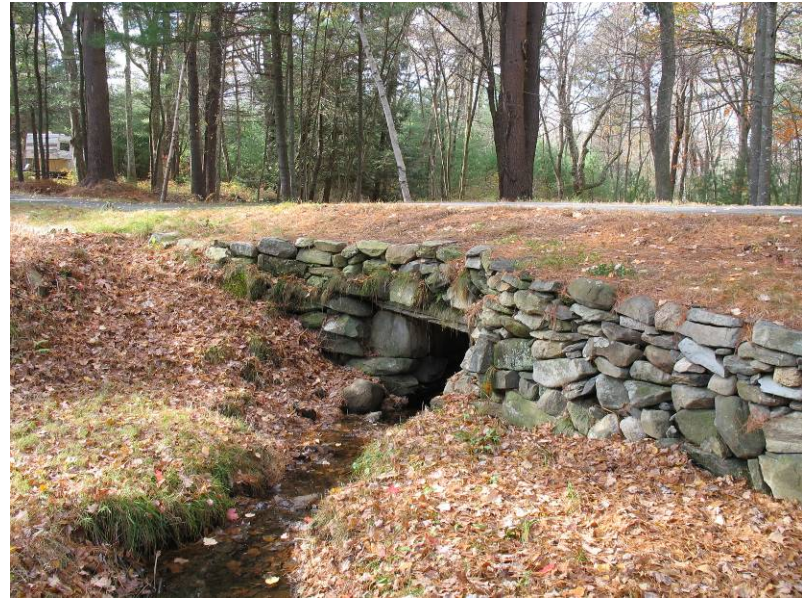
Photo 6: View of private driveway with culvert about 50 ft downstream of the dams' outlet.
