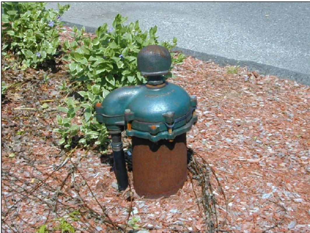
Typical Private Well Photo: Bing.com
