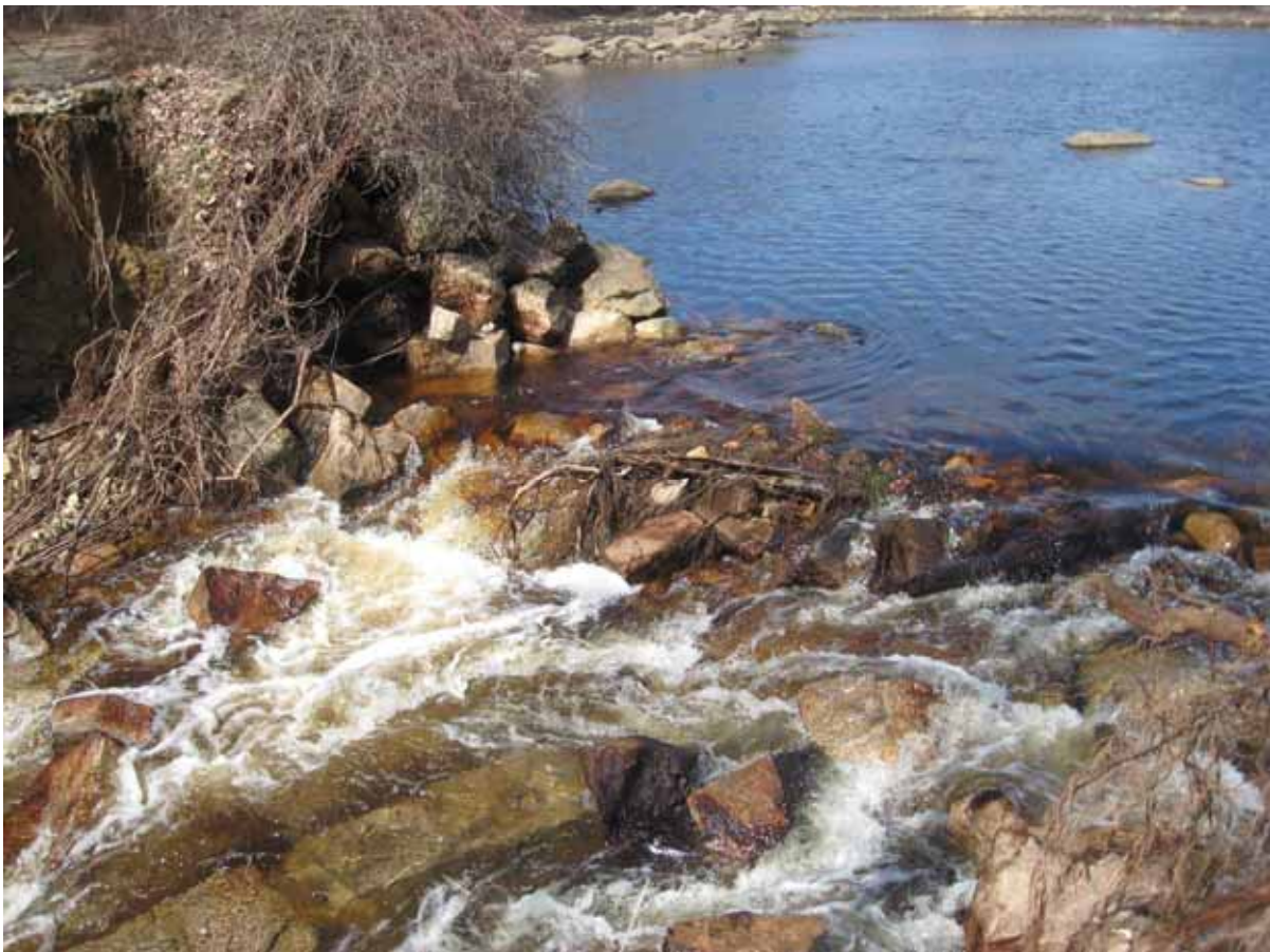
Failed section of Blue Pond Dam (no. 229) in Hopkinton
