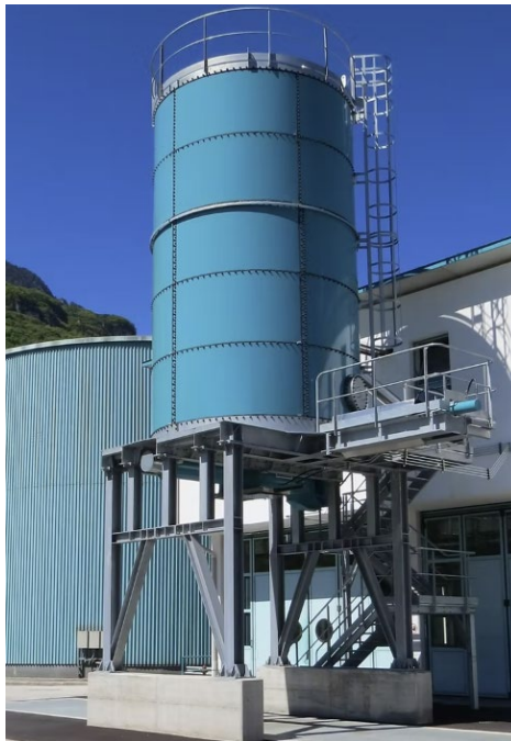
Figure 6 Example of Dried Feedstock Silos
