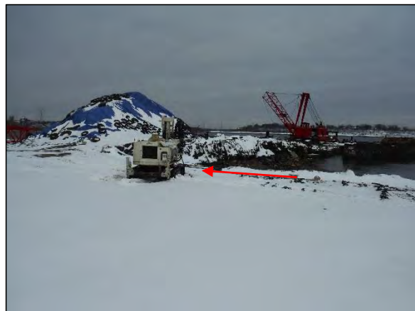
Photo 4 The location of soil boring SB-05/CMW-04, as indicated by the red arrow, during subsurface investigation activities on February 9, 2016, as viewed from the southwest.
