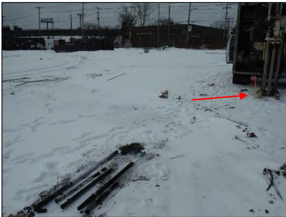
Photo 3 The location of soil boring SB-01/CMW-01, as indicated by the red arrow, during subsurface investigation activities on February 9, 2016, as viewed from the northeast.
