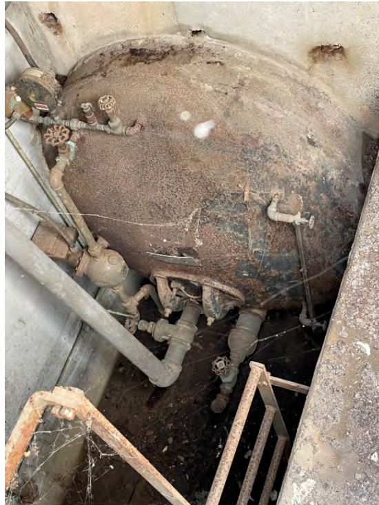
Sub-Grade Infrastructure which Appears to be Associated with a Former Steam Heating System
