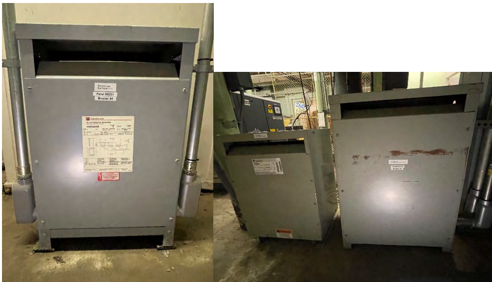
Three (3) Floor-Mounted Transformers Two (2) are labeled as Dry Transformers and One (1) was Unlabeled.
