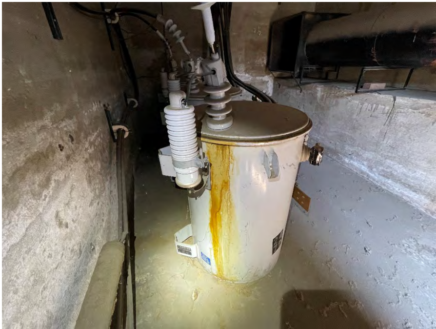
Staining on Exterior of Transformer
