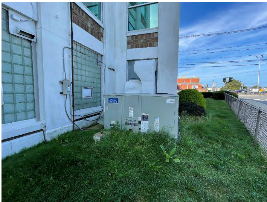
American Standard Natural Gas Forced Air Furnace – North Side of Building
