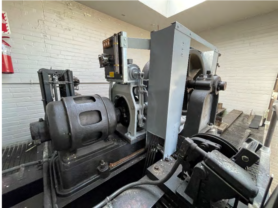
Freight Elevator – Machine Room
