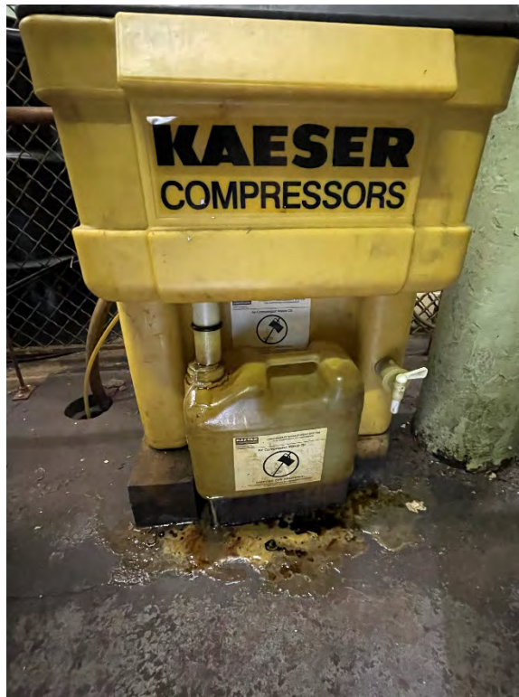
OWS - Waste Oil on the Concrete Floor and Floor Drain Located Behind the OWS
