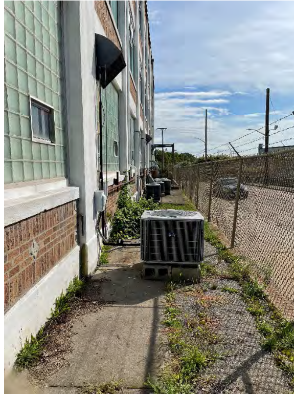
Condensers – South Side of Building
