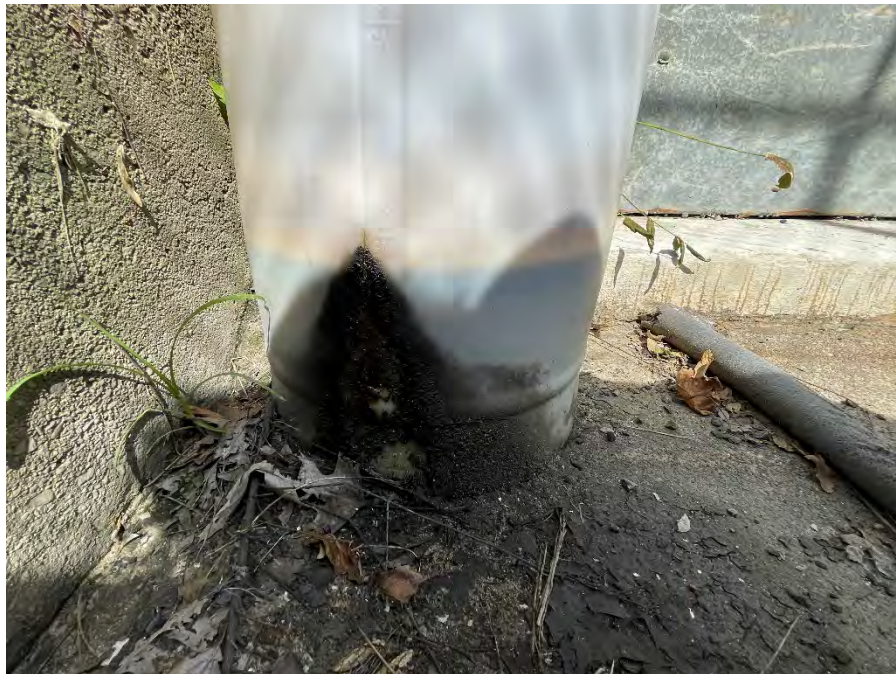
Condensate Collection Container – Approximate 15-Gallon Capacity – Staining on Exterior
