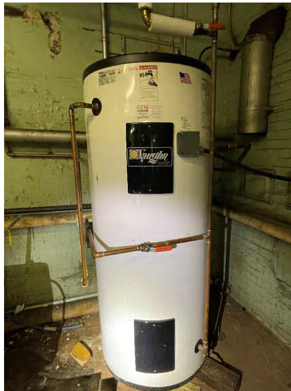
Hot Water Maker
