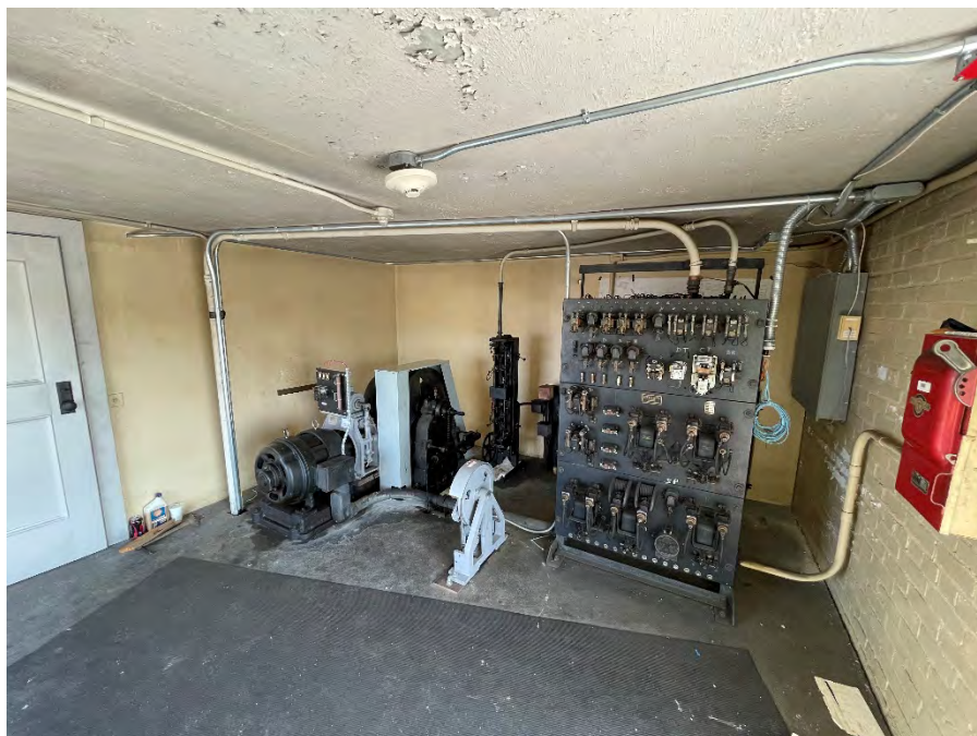
Machine Room – Passenger Elevator
