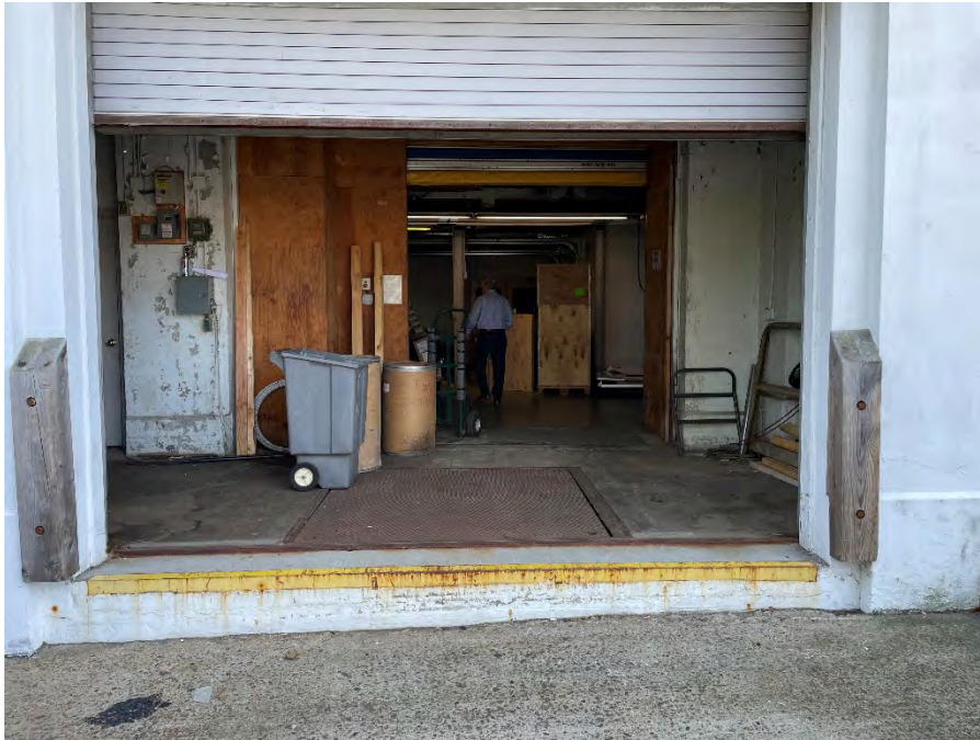
Representative View of Loading Dock – Hydraulics Inaccessible at Time of Site Walkover
