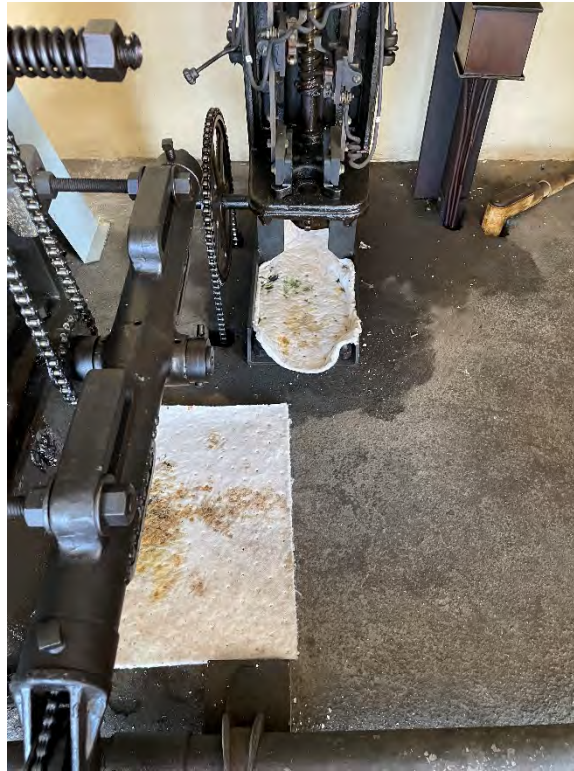
Absorbent Pads – Passenger Elevator Machine Room
