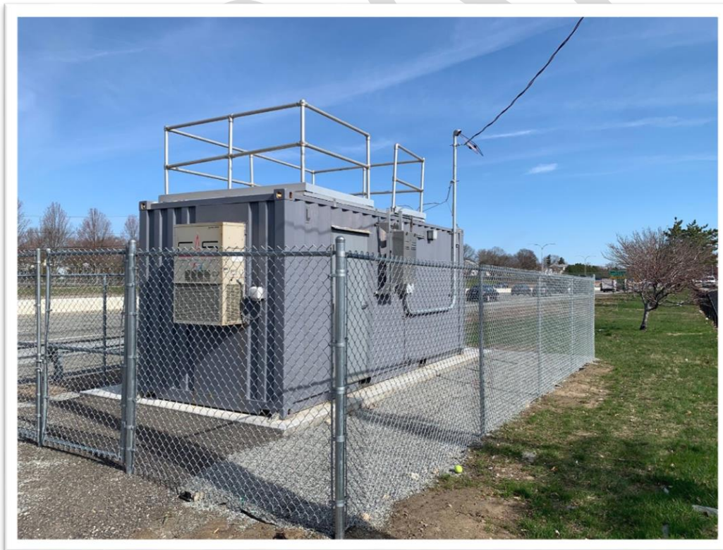
Figure 12: New Cranston Near-Road Monitoring Location (facing NW)
