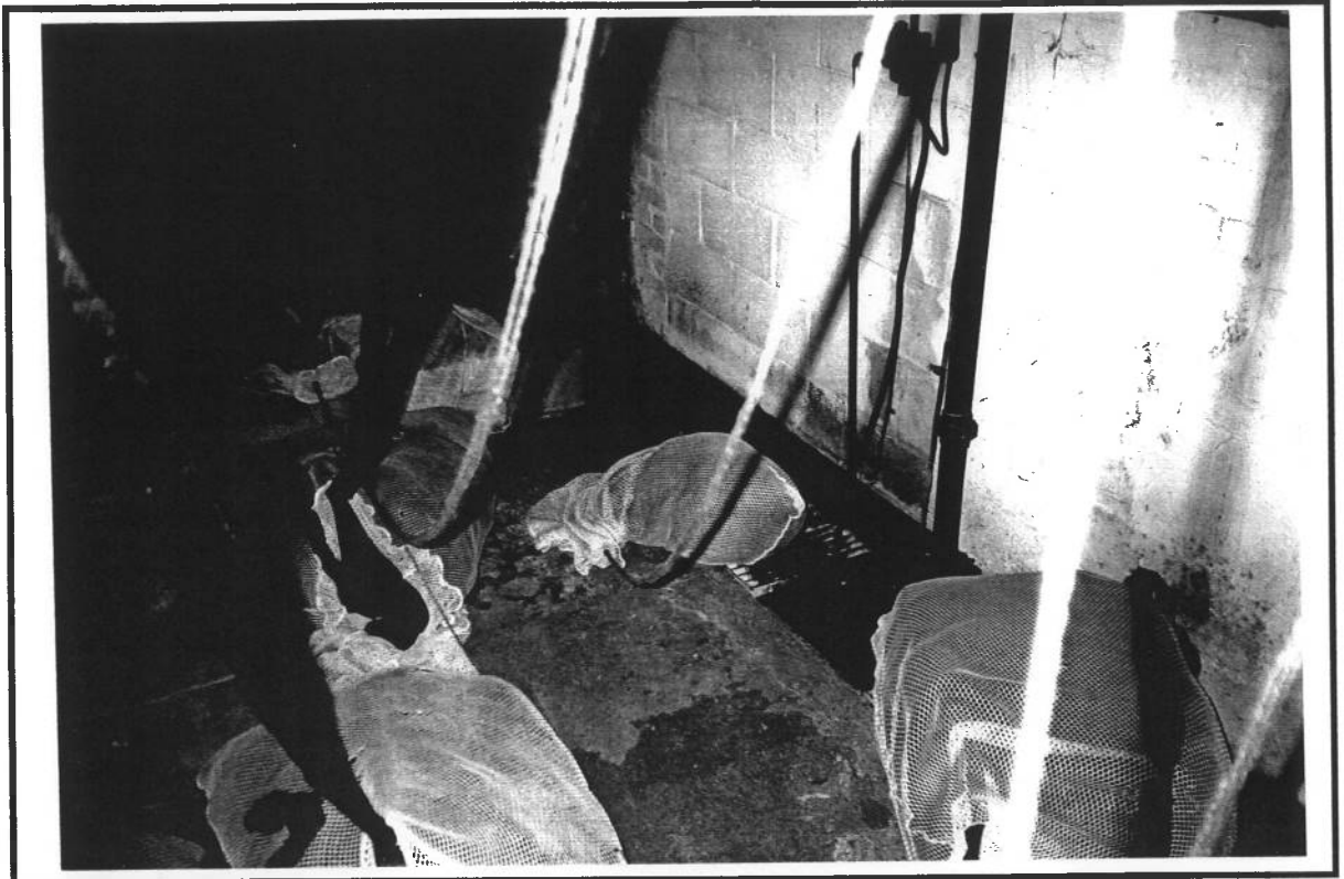
Photo No. 13: Sump pump.
