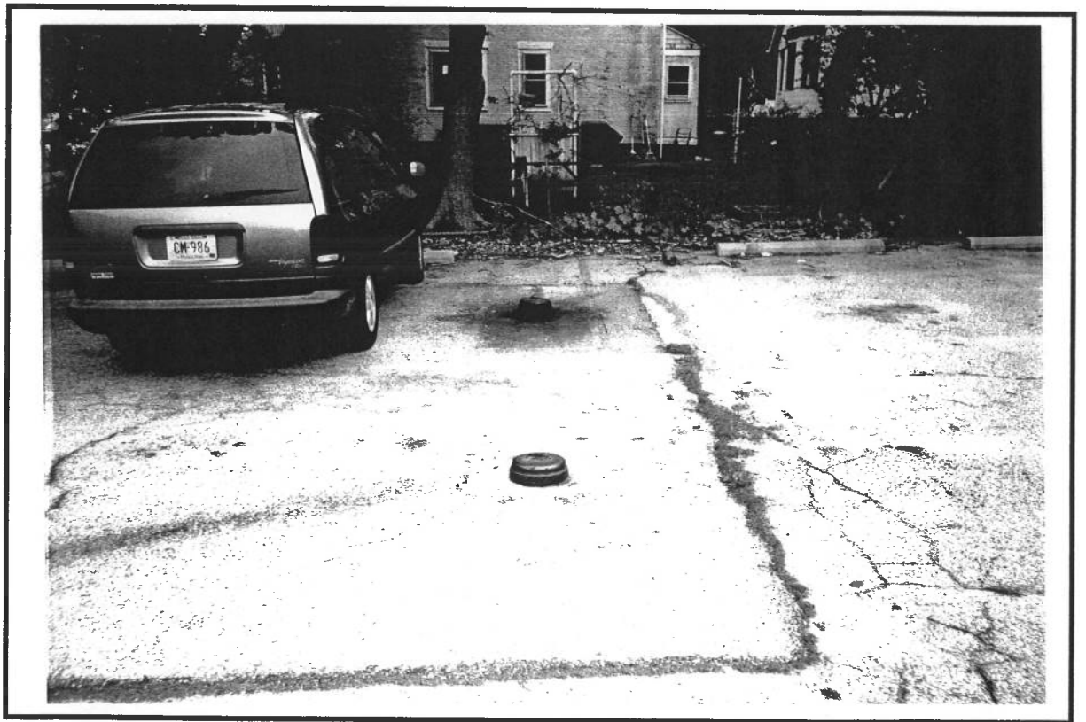
Photo No. 2: View of oil fill ports and footprint of 20,000-gallons of No 6 heating oil USTs.
