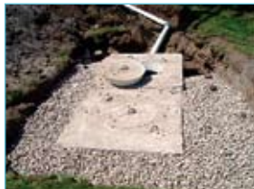
Installed infiltration chamber
