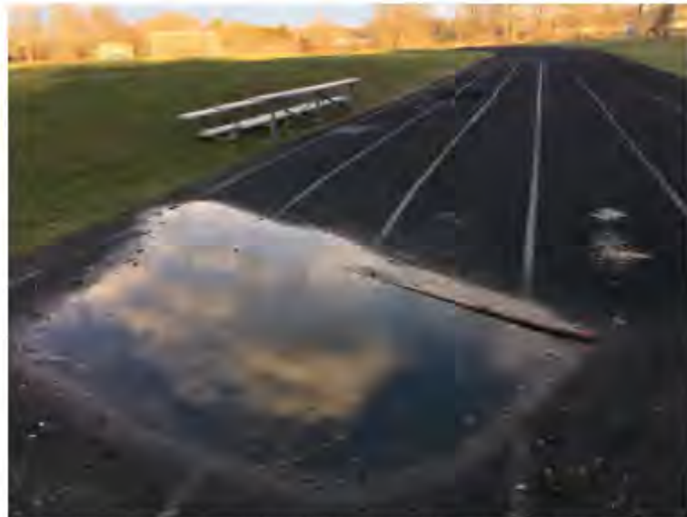
The new athletic field at Rogers High School in Newport is plagued by settlement issues and insufficient drainage.
