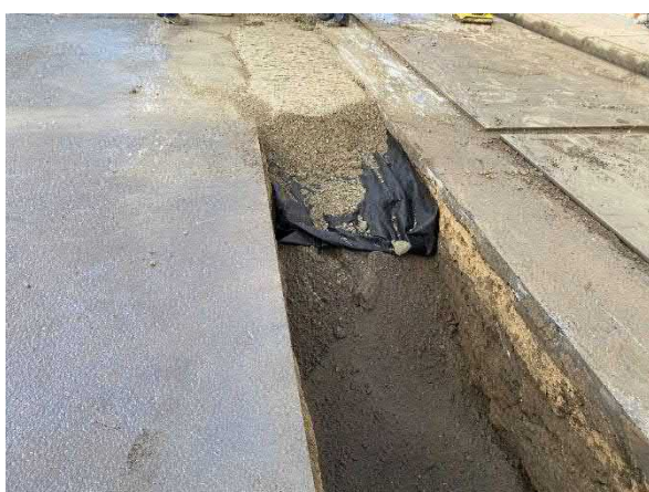
Picture 8: Discharge piping backfilled with native soil to within 12 inches of the surface, geotextile fabric for demarcation, and clean backfill material to grade.
