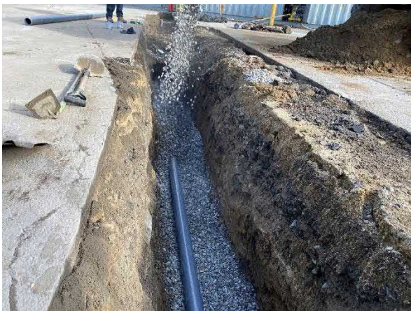
Picture 5: Strategic using peastone to backfill around the discharge pipe in front of the remediation trailer.
