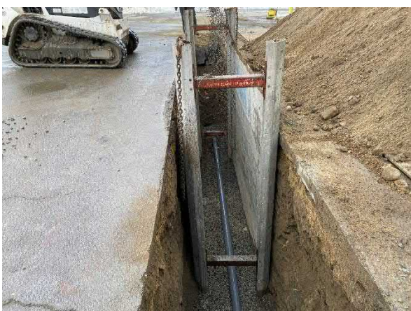
Picture 7: Installation of discharge piping along the western side of the building.
