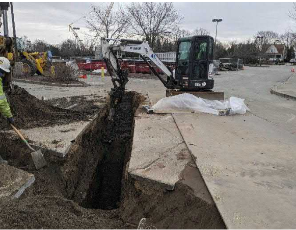
Picture 11: Strategic hammering hardpan material in trench near the front of the building.
