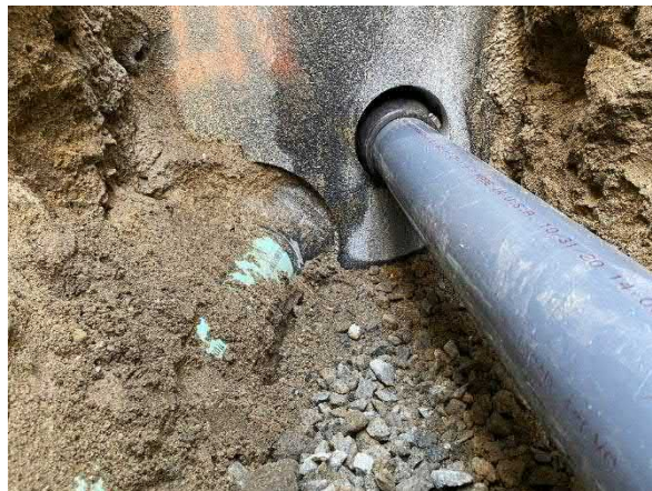
Picture 18: Final connection of the effluent discharge piping to the sewer manhole.
