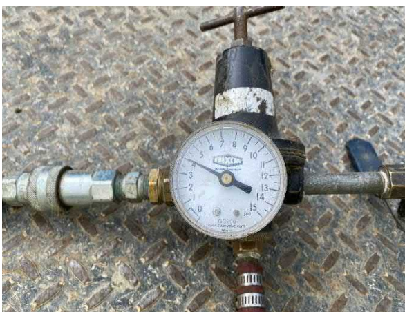
Picture 19: Picture of the pressure testing of the effluent discharge piping at 4 psi.
