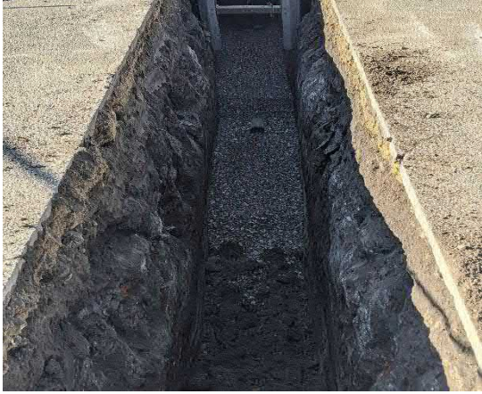
Picture 13: Section of pipe backfilled with pea gravel in trench past the handicap spots.
