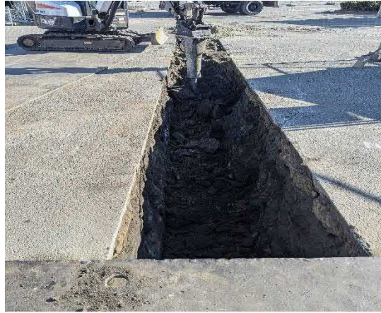
Picture 14: Strategic hammering hardpan material from trench before dogleg to storm drain.
