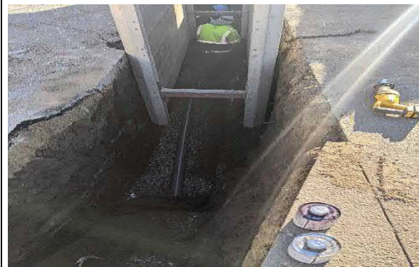
Picture 12: Strategic installing a section of piping near the handicap parking spots.
