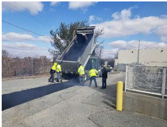
Picture 22: Strategic paving trench line near the remediation trailer behind the building.
