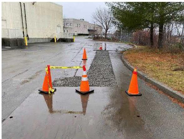
Picture 6: Trench in front of remediation trailer backfilled and compacted to grade with clean backfill material.
