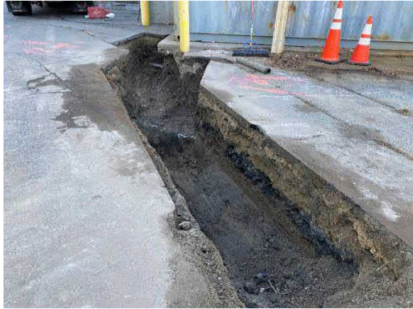
Picture 2: Strategic beginning to excavate trench in front of the remediation trailer.
