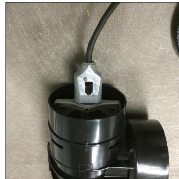
Float switch installed in effluent screen
