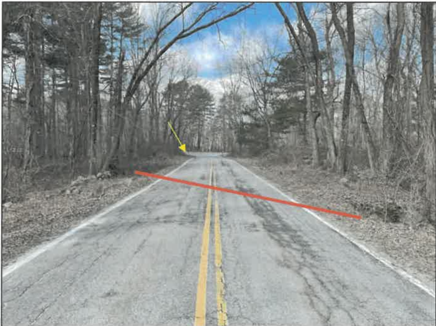
Photo No. 10.: View of Central Avenue located downstream of the dike embankment. Note the alignment of the culvert crossing along Central Avenue (red line) in the foreground and the location of the Route 116 culvert crossing (yellow arrow) in the background
