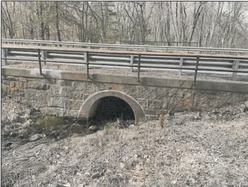
Photo No. 12.: Upstream end of the Route 116 culvert crossing located downstream of the dike.
