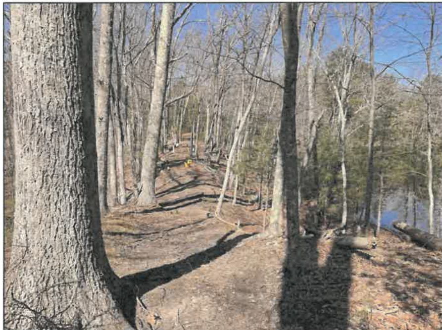
Photo No. 8.: Shoestring Mill Dike embankment from the left abutment looking right.
