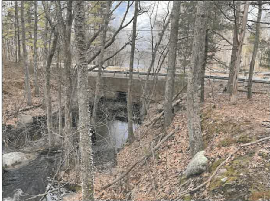
Photo No. 7.: View of the Route 116 culvert crossing downstream of the former Shoestring Mill Pond Dam site.
