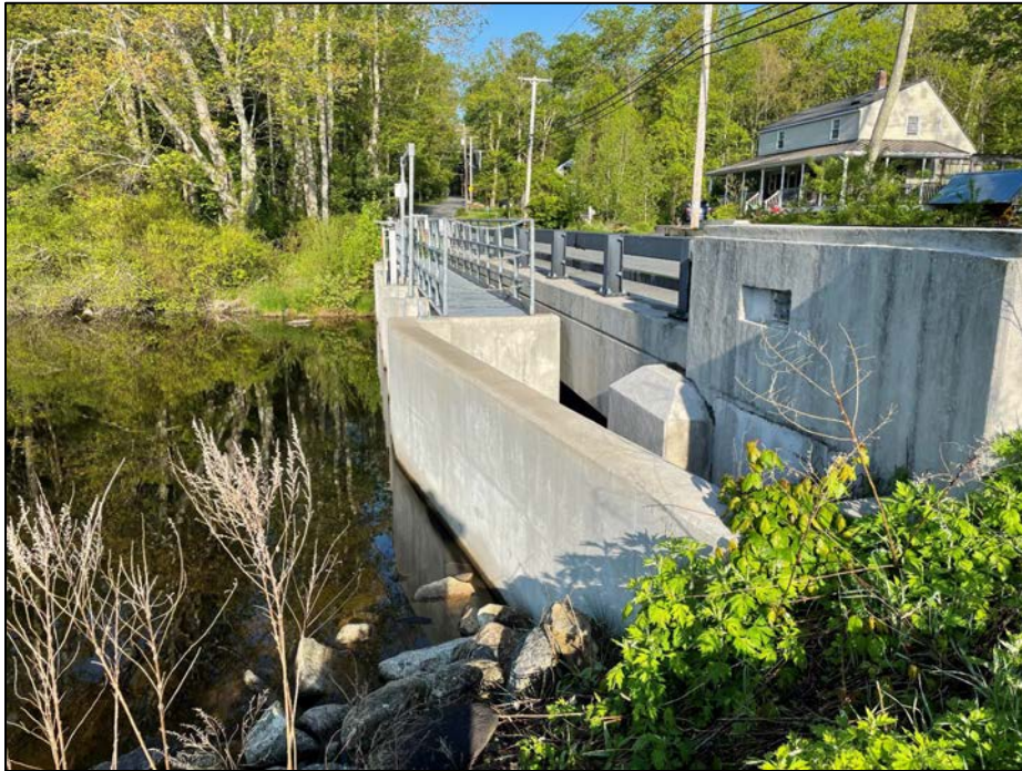
Photo No. 17.: Spillway approach and controls section from the right end looking left.
