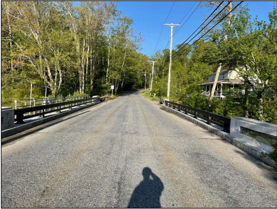
Photo No. 6.: Crest from right of the bridge over the spillway channel looking left.
