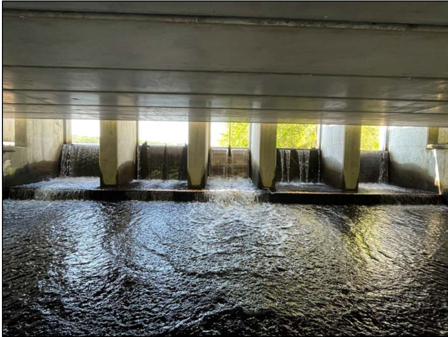
Photo No. 19.: View of the five control bays of the spillway; all bays are stop log controlled except for the upward operating slide gate within the center bay.
