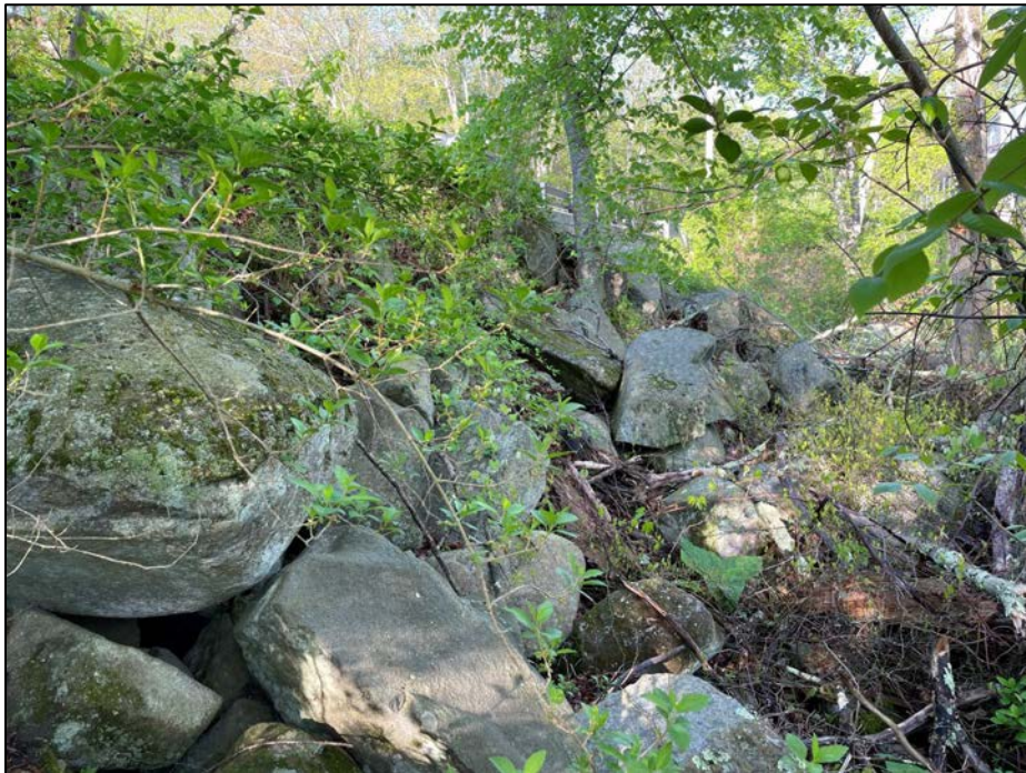
Photo No. 10.: View of the large and irregularly stacked boulders of the downstream slope looking left.
