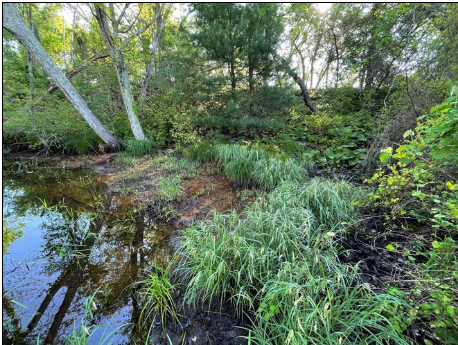
Photo No. 14.: View of the saturated downstream area with iron oxide staining and low flow along the toe of the right abutment slope.
