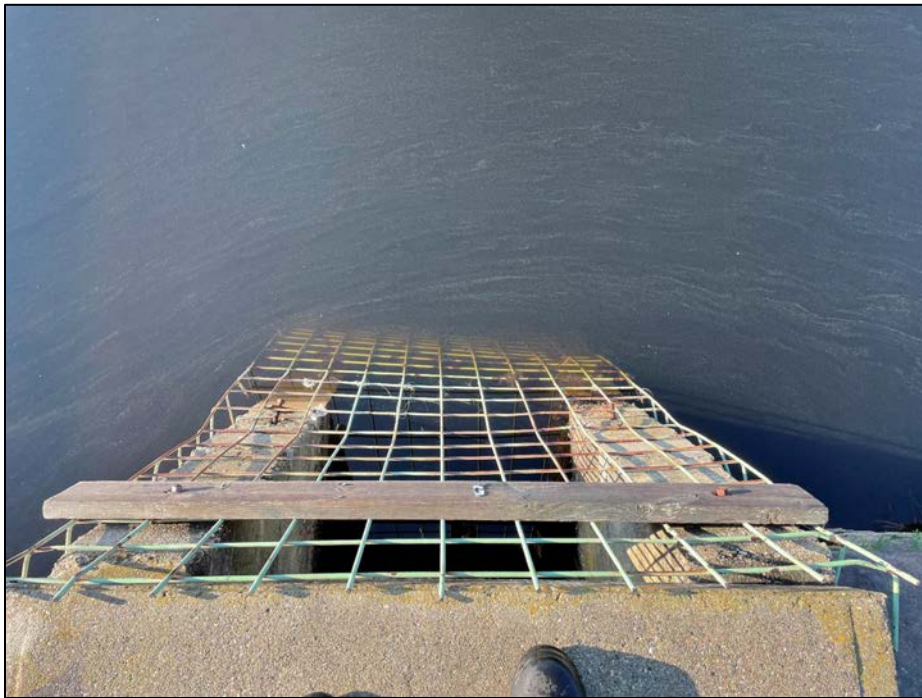
Photo No. 25.: Trash rack at the upstream end of the intake structure.
