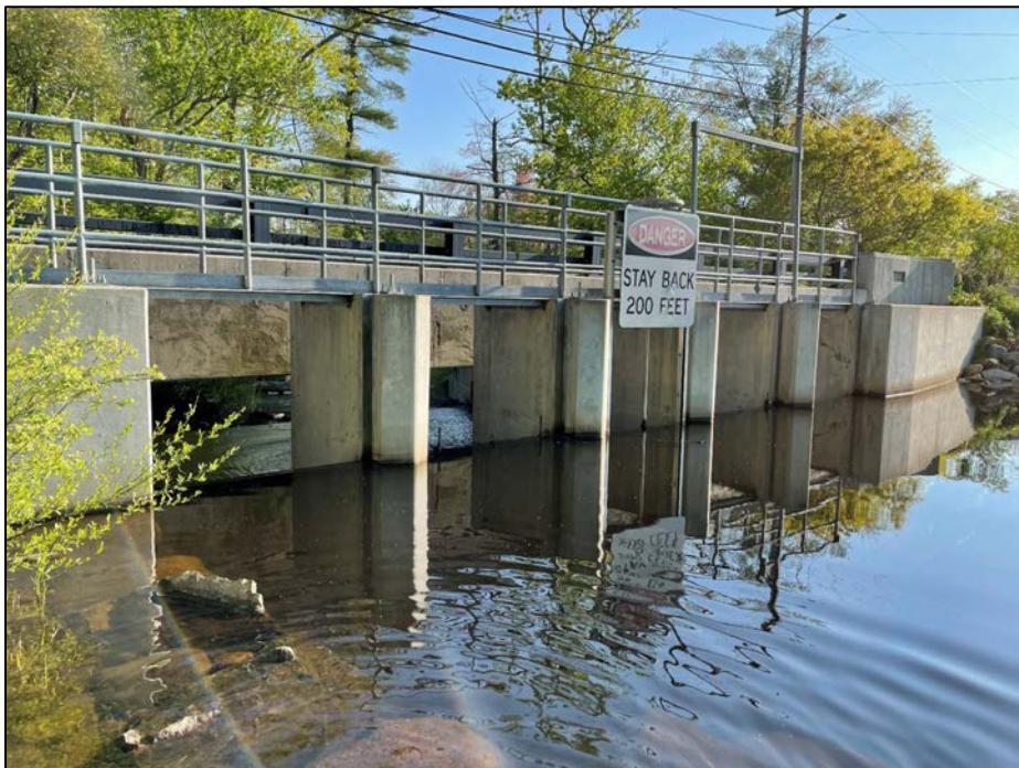
Photo No. 16.: Approach and upstream side of the controls of the spillway system.
