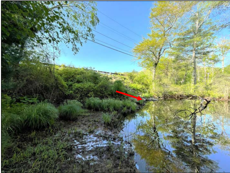
Photo No. 13.: View of the downstream slope from the right edge of the tailwater pool looking left and upstream. Note location of the LLO pipe (red arrow). Note the tall tree growth along the left (photo right) half of the slope and smaller height weed and brush growth along the right half (photo left)
