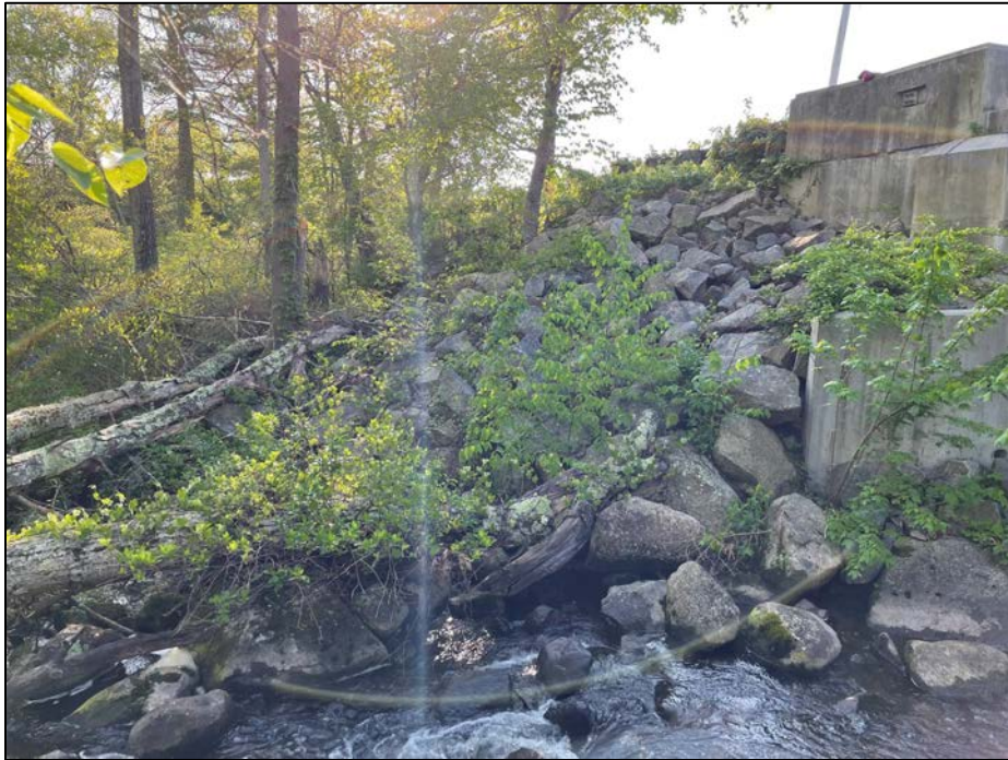
Photo No. 9.: Downstream slope from the spillway channel looking right. Note growth of woody vegetation within riprap and along the slope further right.
