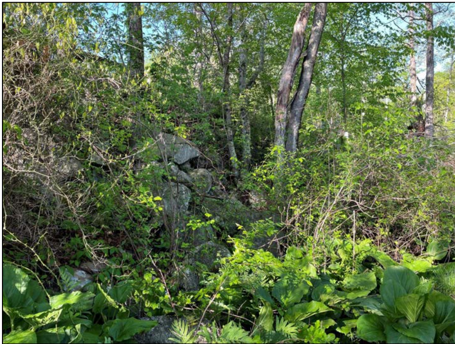
Photo No. 11.: View of the large and irregularly stacked boulders of the downstream slope looking left.
