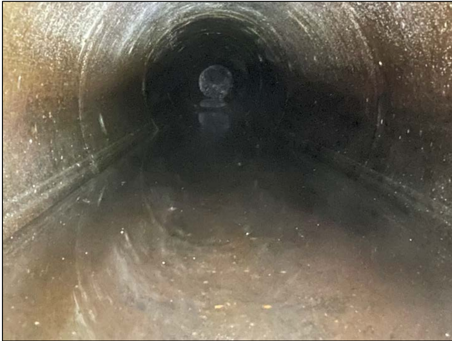
Photo No. 27.: View within the outlet pipe from the outlet end of the pipe looking upstream.
