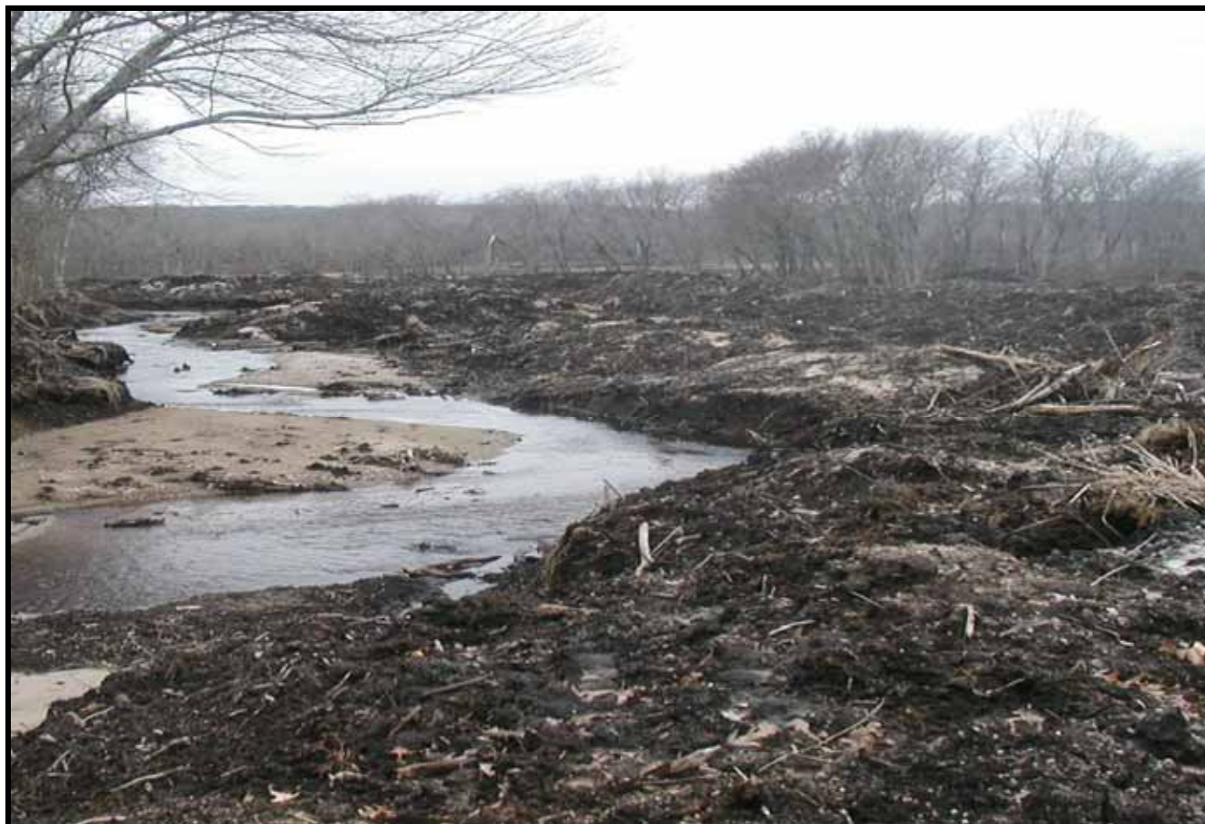
Excavation of about 6.0 acres of a swamp/marsh/stream complex and disposal of the spoils within the wetlands
