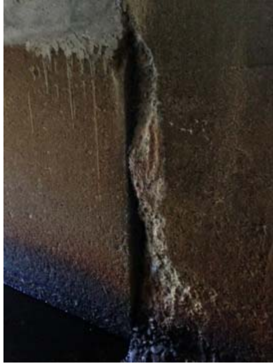
Photo 19: Cracking at first joint in concrete culvert at primary spillway
