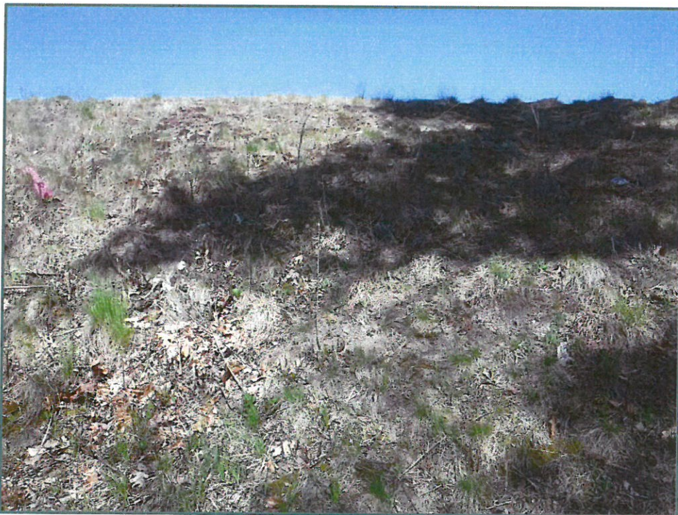
Photo No. 12: Typical sparse grass cover along the downstream slope of the north embankment, looking west, photo taken on May 11, 2020.
