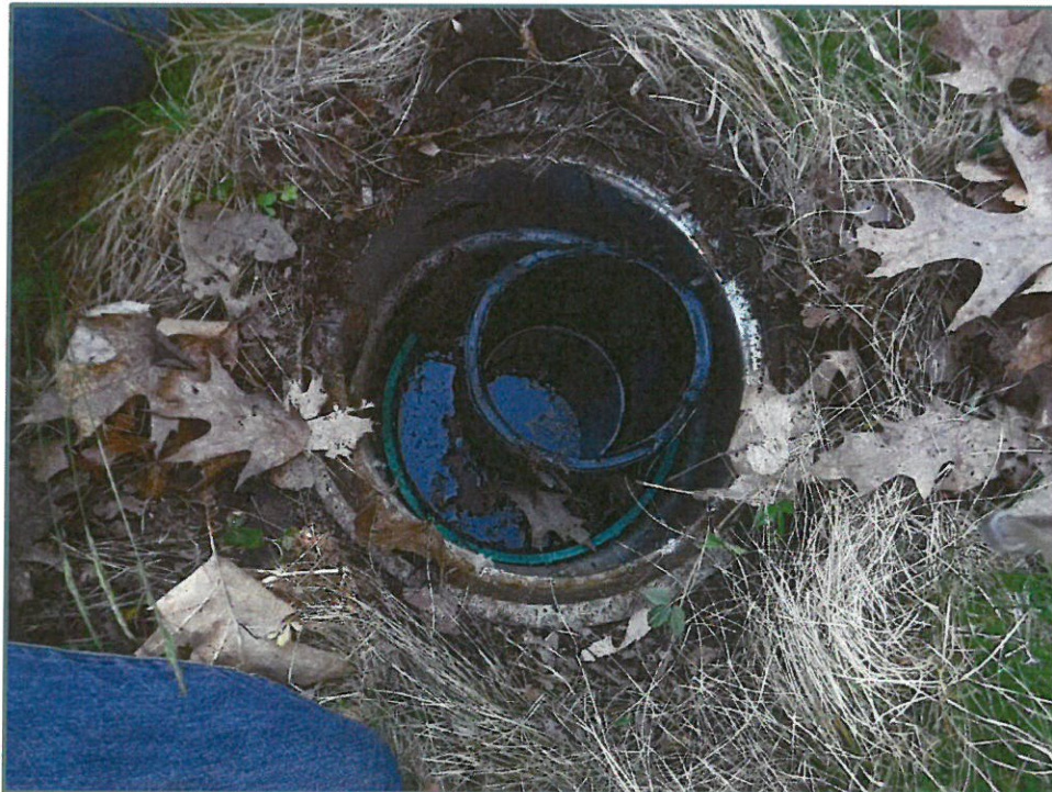
Photo No. 26: Standing water within the secondary toe-drain cleanout, looking down, photo taken on May 11, 2020.
