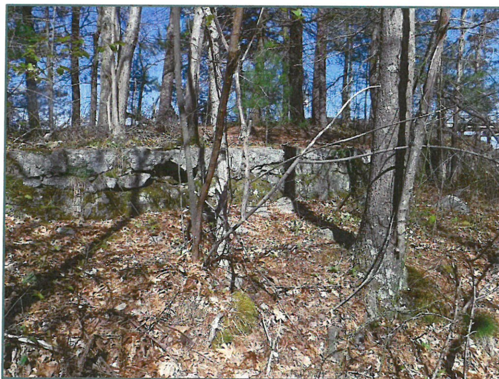
Photo No. 10: Voids within and heavy vegetation at the downstream masonry training wall, looking southwest, photo taken on May 11, 2020.
