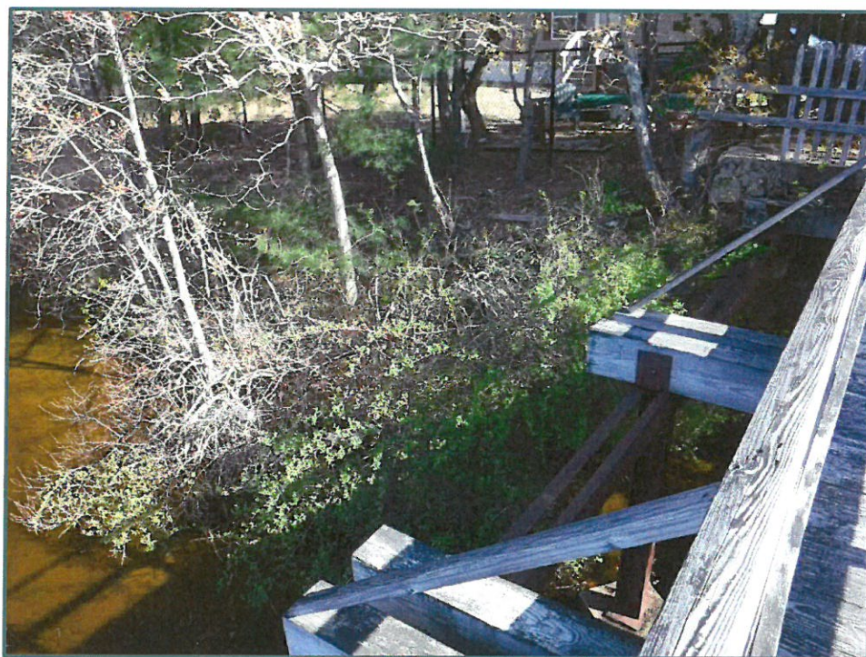
Photo No. 6: Overgrown vegetation along the left side of the upstream spillway area, looking north, photo taken on May 11, 2020.
