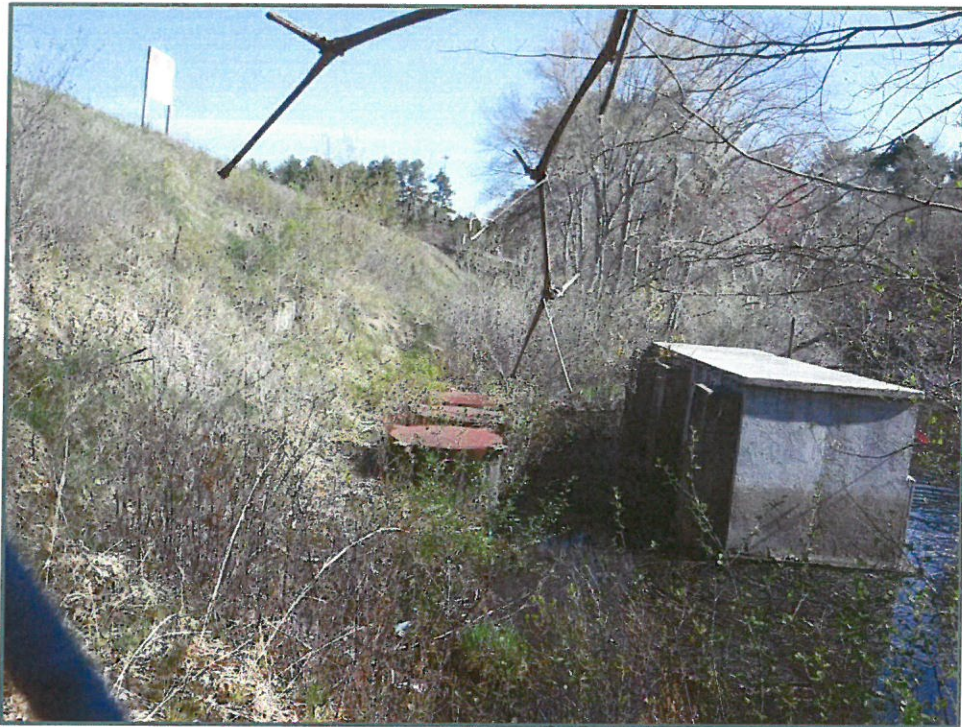
Photo No. 19: Thick woody vegetation near the downstream outlet structure, looking north, photo taken on May 11, 2020.
