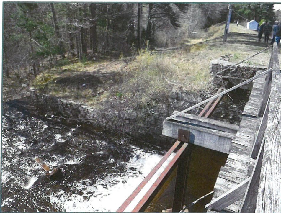
Photo No. 5: Overgrown vegetation behind the south abutment wall, looking south, photo taken on May 11, 2020.
