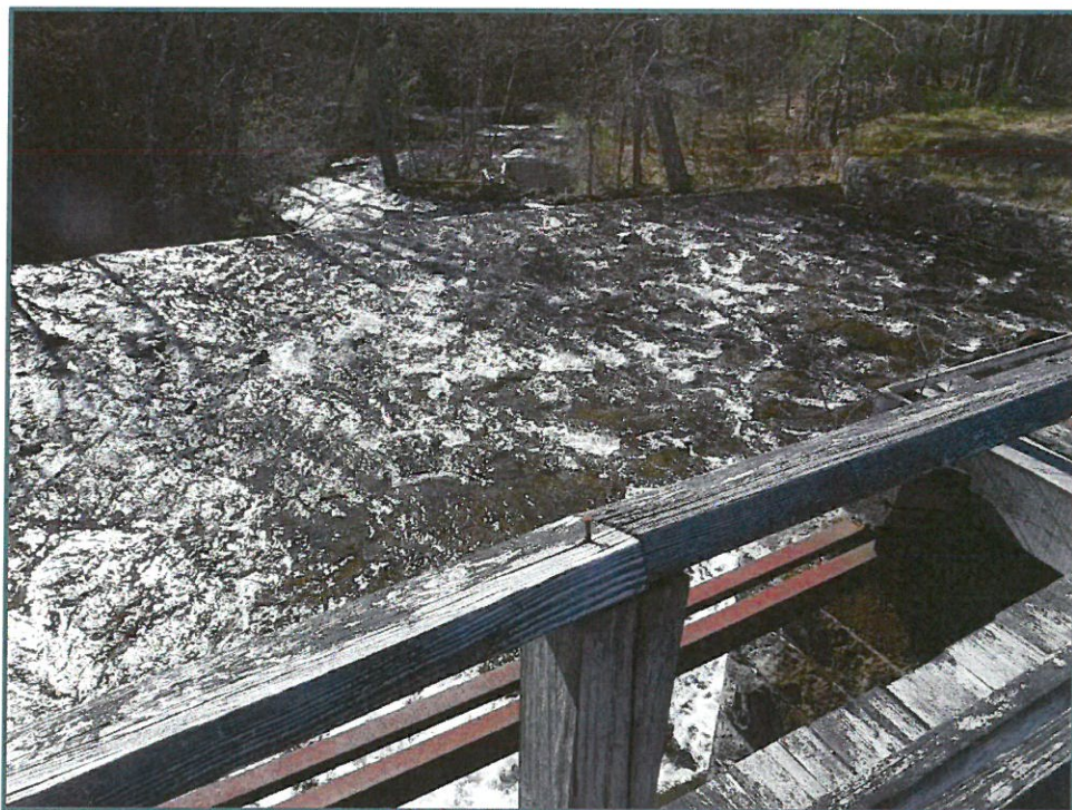
Photo No. 8: Loose timber handrail and fastener along the timber footbridge, looking southeast, photo taken on May 11, 2020.
