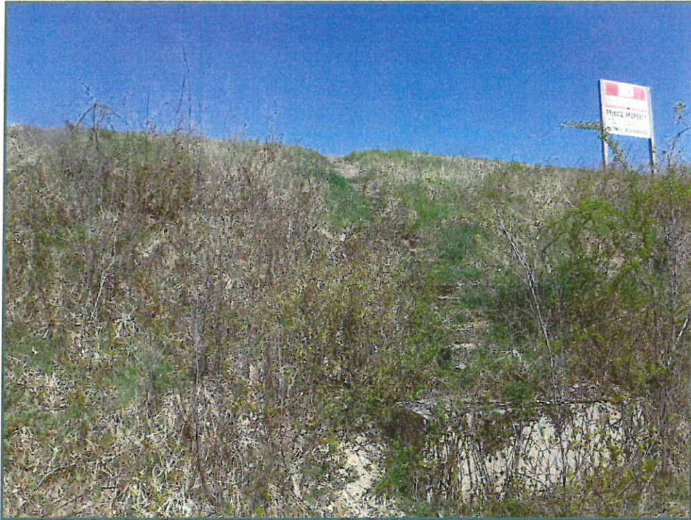
Photo No. 15: Overgrown woody vegetation along the downstream slope of the north embankment, looking west, photo taken on May 11, 2020.
