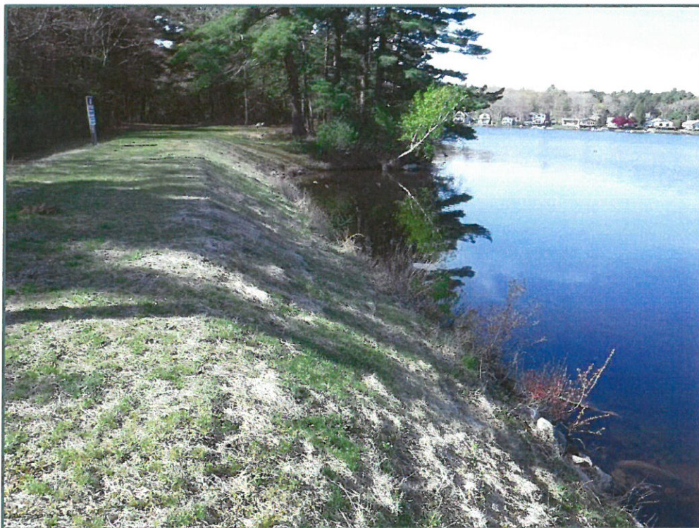
Photo No. 16: “Test Section” at the crest and upstream slope of the north embankment, looking southwest, photo taken on May 11, 2020.
