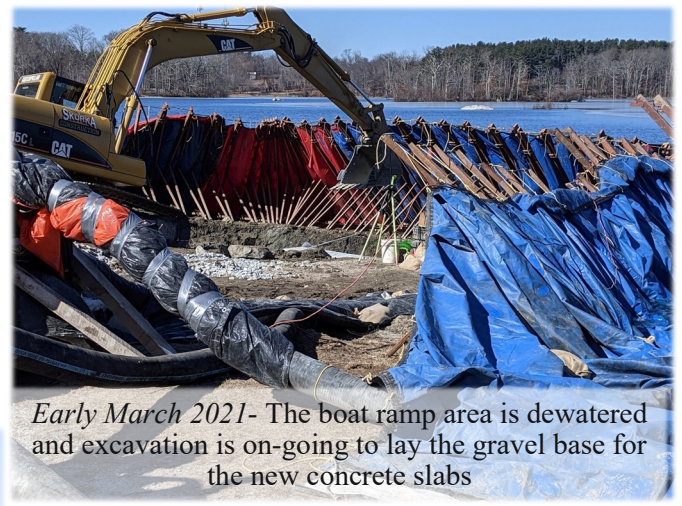
Early March 2021- Setting up the Portadam to dewater the area for the new boat ramp. Portadam had to chip through about 8 in. of ice on Olney Pond to get this installed.
