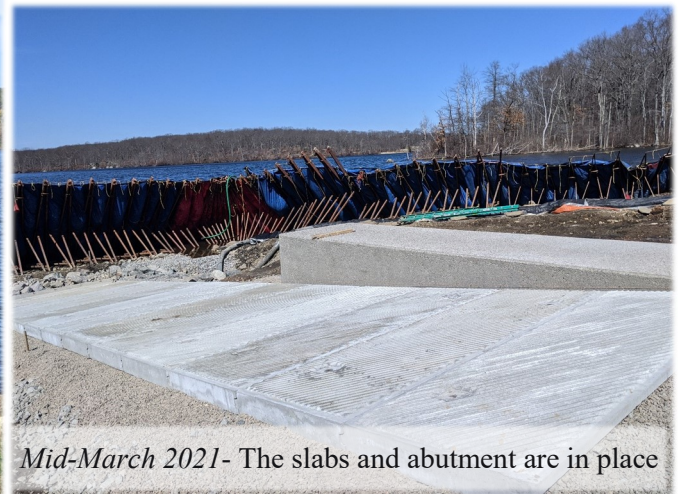
Early March 2021- The boat ramp area is dewatered and excavation is on-going to lay the gravel base for the new concrete slabs
