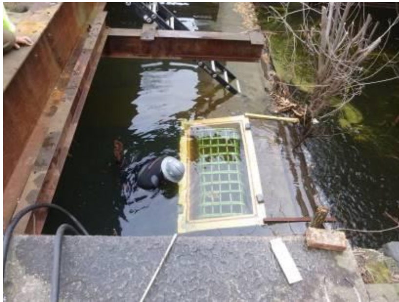
Bleachery Pond Dam (No. 104) in Lincoln, undergoing repair without lowering the pond
