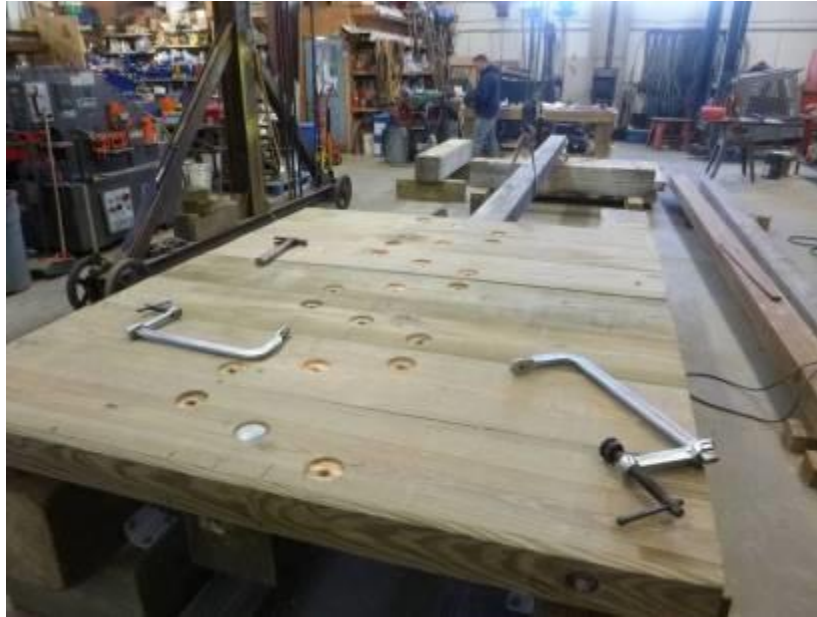
Fabrication of new low level outlet gates for the Flat River Reservoir Dam (No. 167) in Coventry
