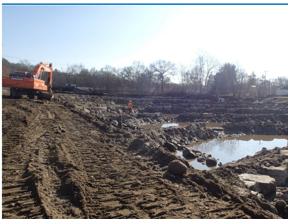
Bradford Construction- weirs with low flow outlets. Photo courtesy of P. Edwards
