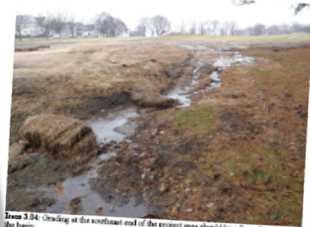
Item 3.03: Ertel has been grading to end of the concrete level spreader to prevent runoff from bypassing the spreader. Repair existing erosion gullies and stabilize with riprap or crushed stone.
