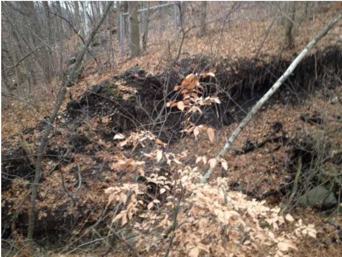
12/16/14 - View of the south wall of the washout.
