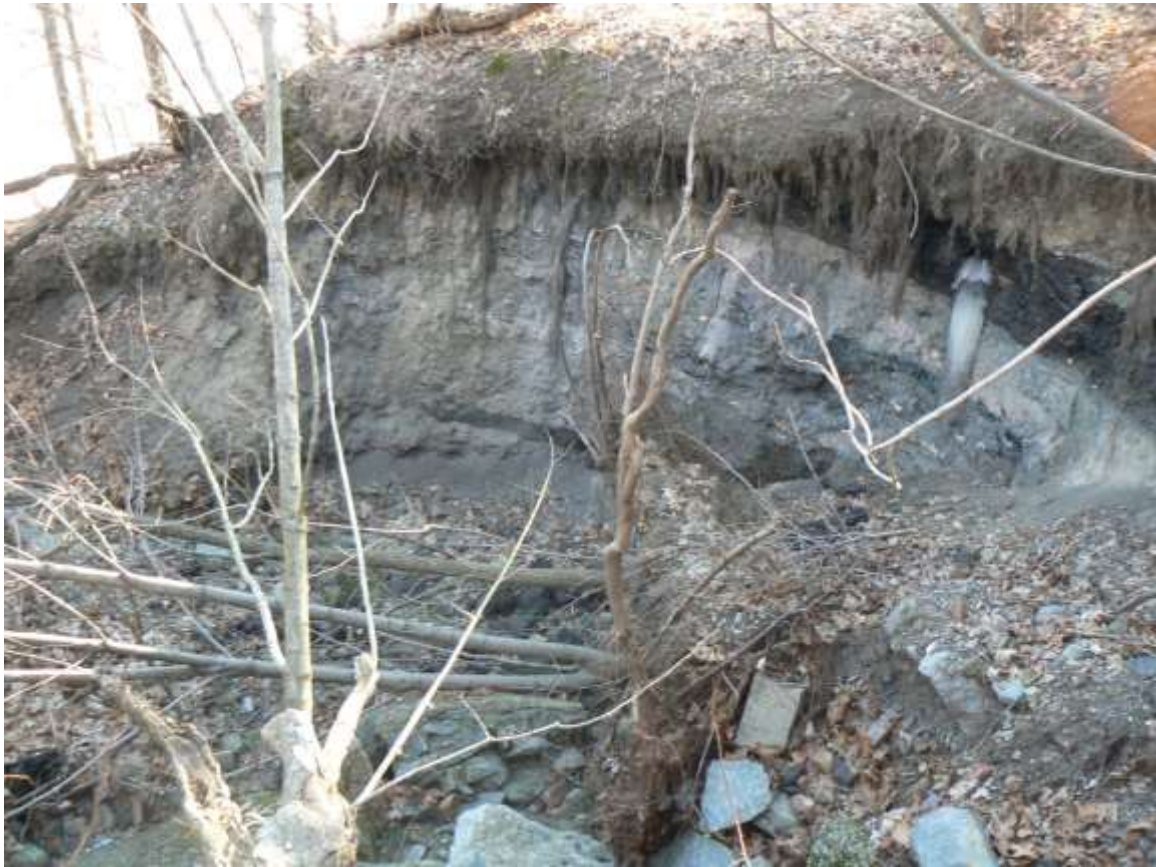
View of the washout, as seen from the top of the northern wall.
