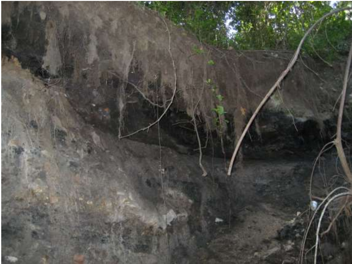
View of the south wall of the washout.
