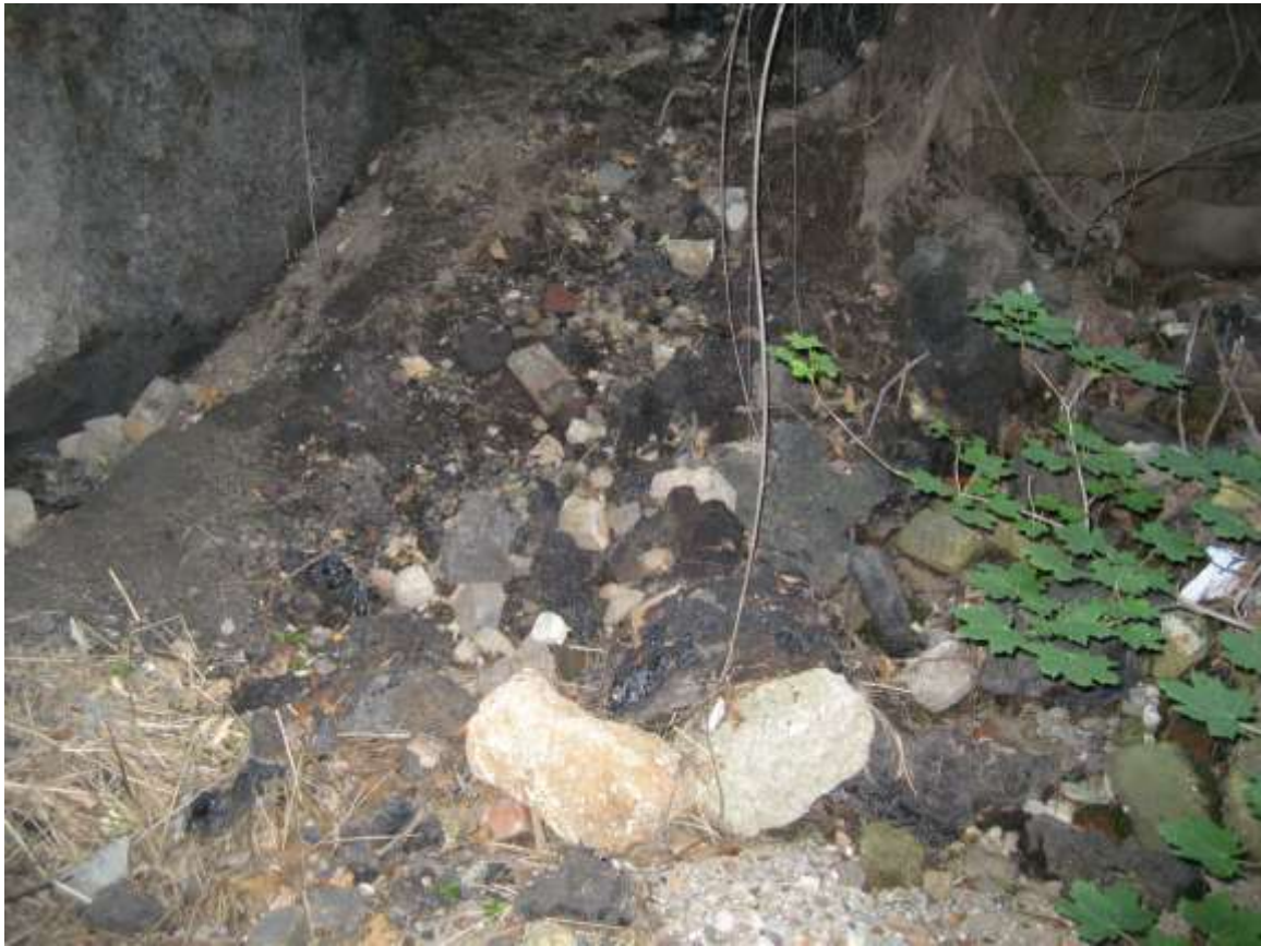
View of the washout area from inside the washout.
