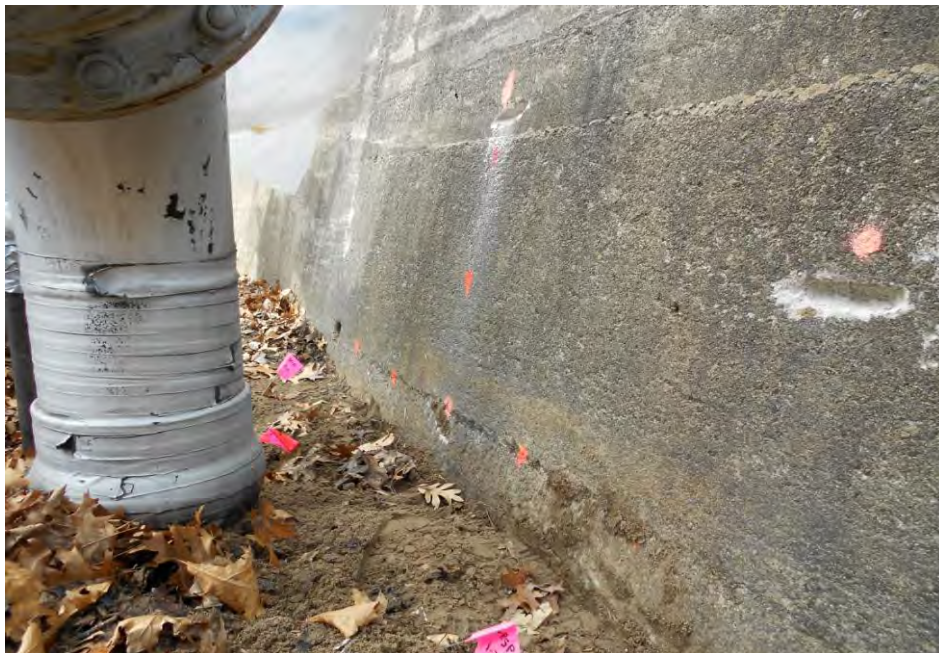
Closeup of impacted soils and retaining wall, April 22, 2011.
