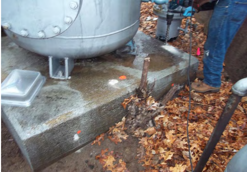
PCB Impacted concrete pad with former scrubber equipment. April 5, 2011.
