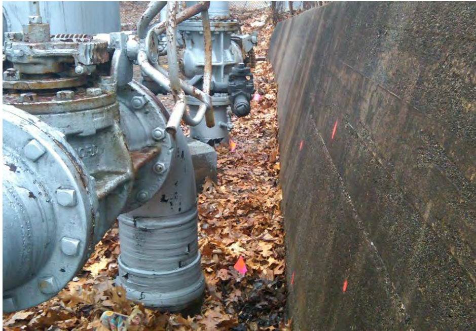
Area of former leaky valve and impacted retaining wall, April 5, 2011.
