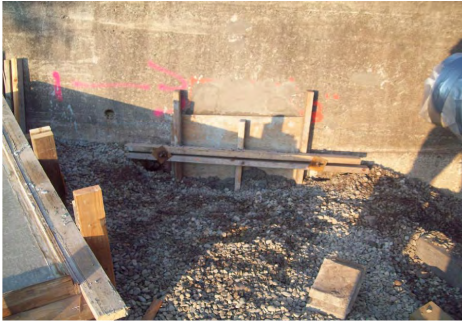
Crushed stone placement over excavated area with retaining wall in foreground. September 14, 2011.
