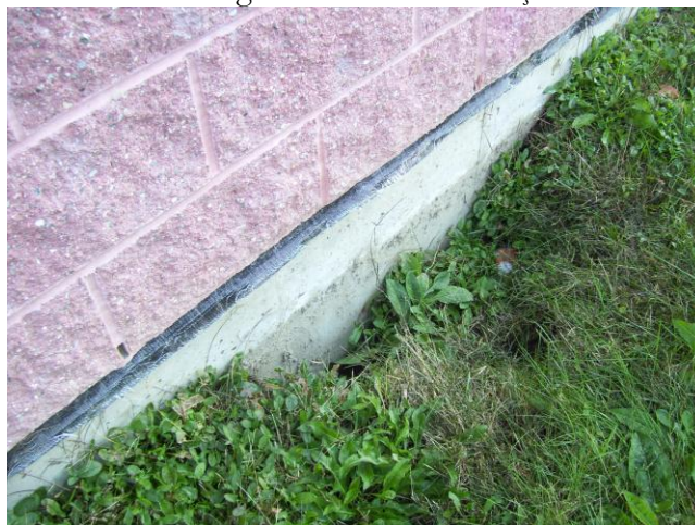
Cavity within cap thickness adjacent to middle school foundation
