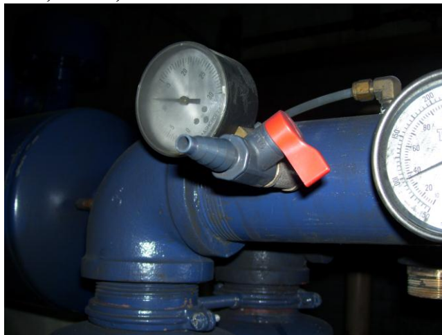
Influent sample port of sub-slab ventilation system
