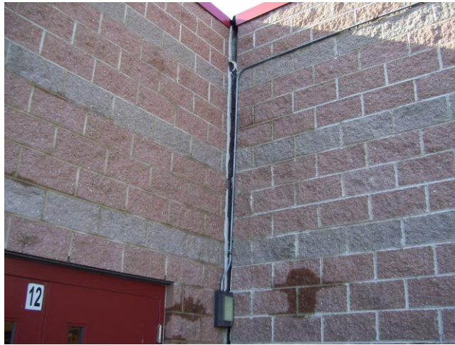
Gap between blower shed and main elementary school building
