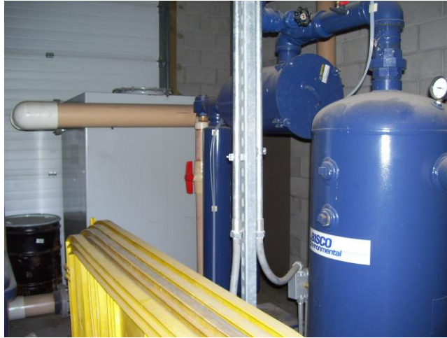
Water tank, blower, carbon vessel of sub-slab ventilation system
