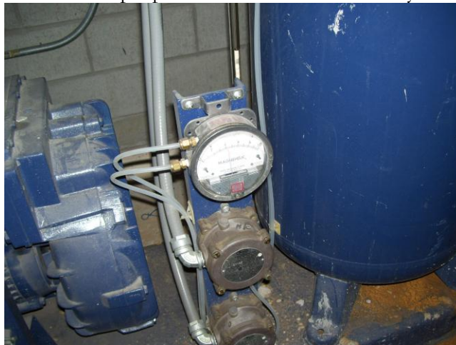
Vacuum gauge of sub-slab ventilation system
