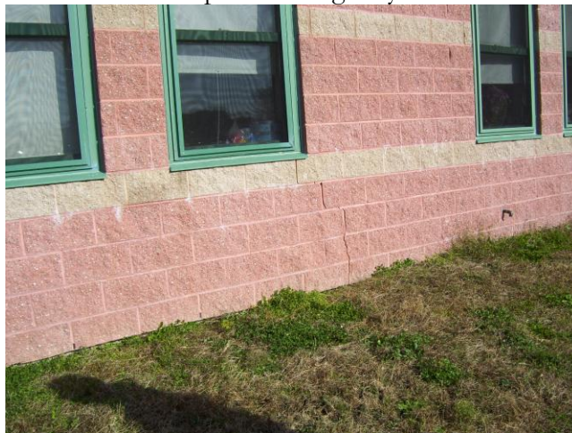
Cracking in middle school façade
