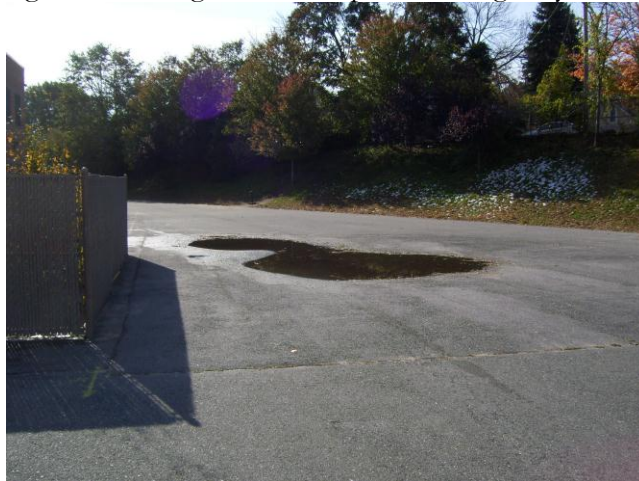
Standing water on pavement behind elementary school
