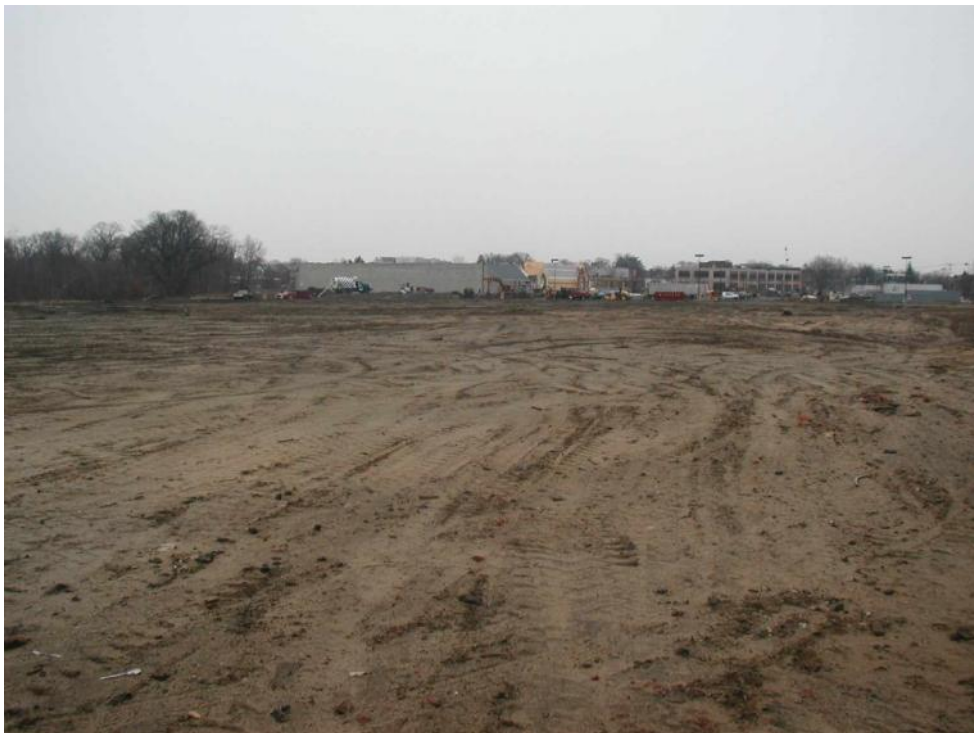
Photo 22. View east from southwest corner of site after final backfill and demobilization.
