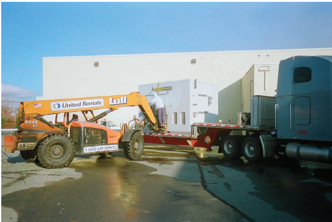
ASD System Enclosure Delivery
