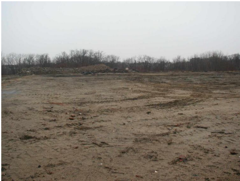
Photo 20. View north from southwest corner of site after final backfill and demobilization.
