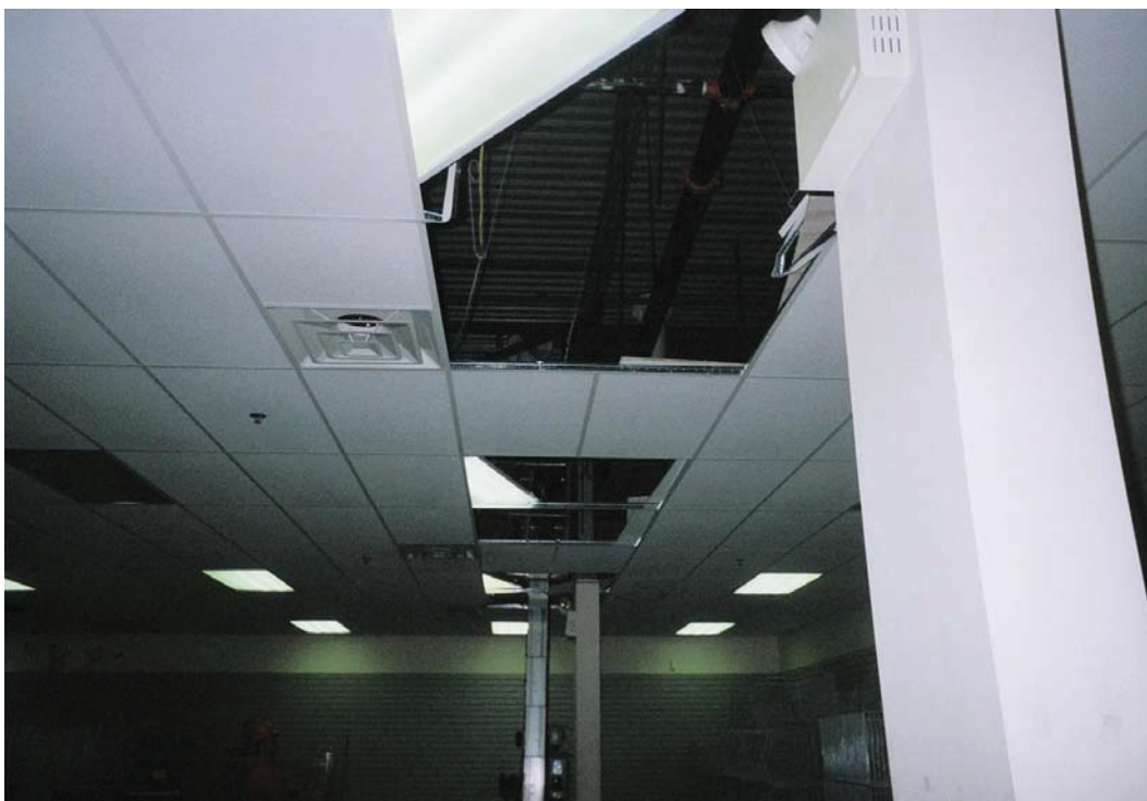
EW-6 Above Drop Ceiling
