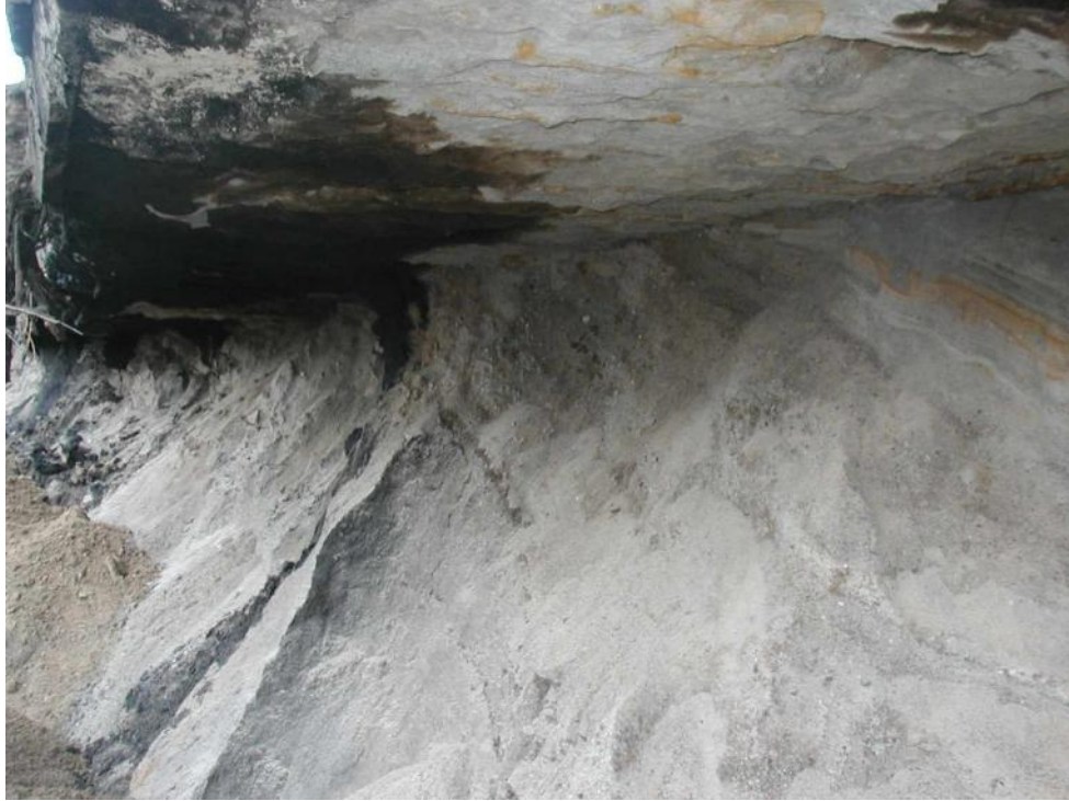
Photo 11. Clean soils directly beneath bunker, with limited staining of underside of bunker floor.
