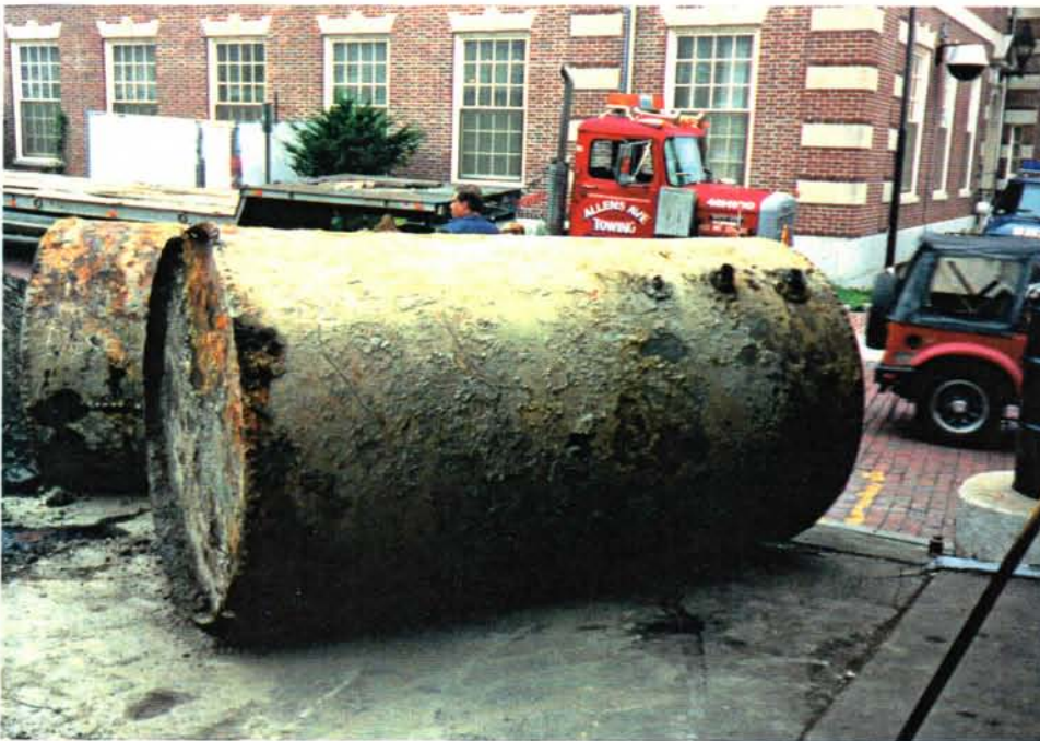
UST #1 1,000 gallon waste oil
