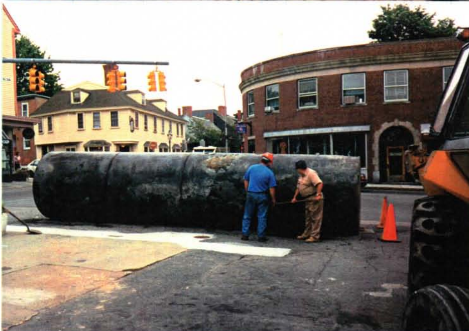
UST #3 4,000 gallon gasoline
