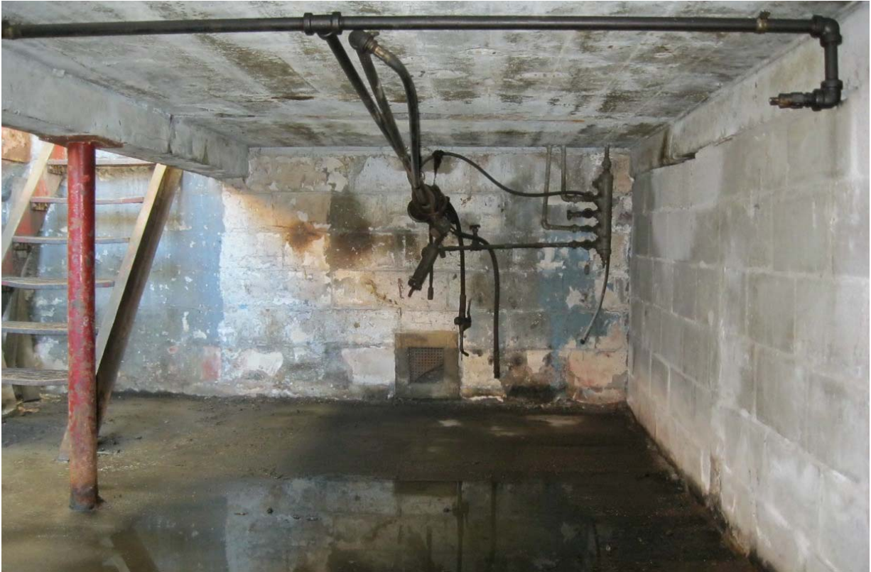
PHOTO 12 : Interior view looking north in the mechanic's pit and sub-floor storage area.
