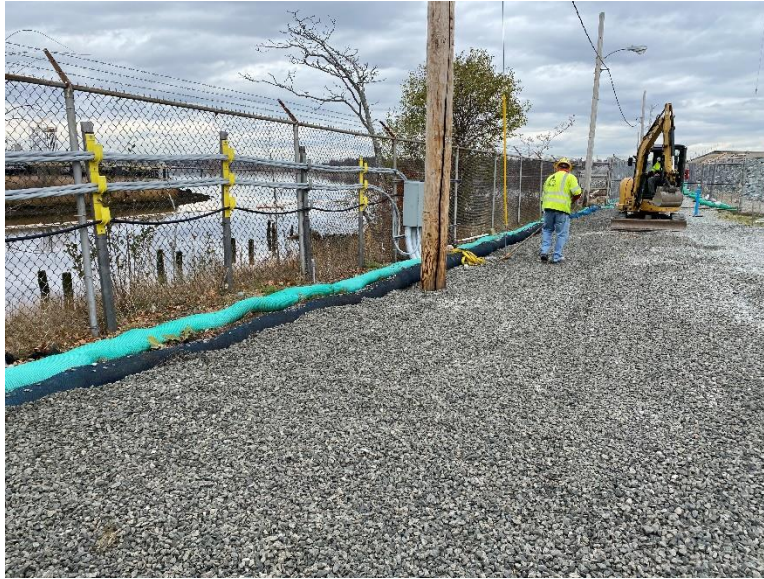
Photo 4: Second row of filtrex soxx on the north side of the access road
