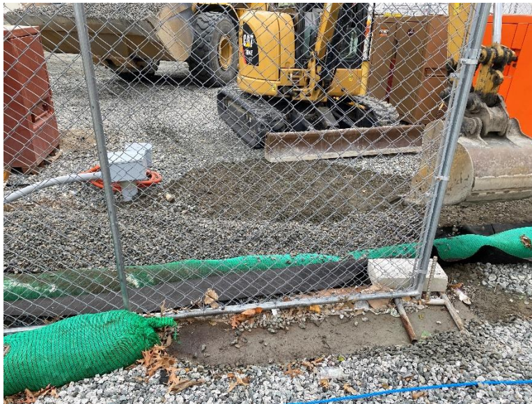
Photo 5: Trench south of steel plates with filter fabric and filtrex soxx, crushed stone added to the area south of the electrical conduit trench.
