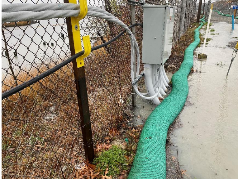
Photo 1: Unanticipated bypass of the perimeter controls on the northern boundary of the Site.
