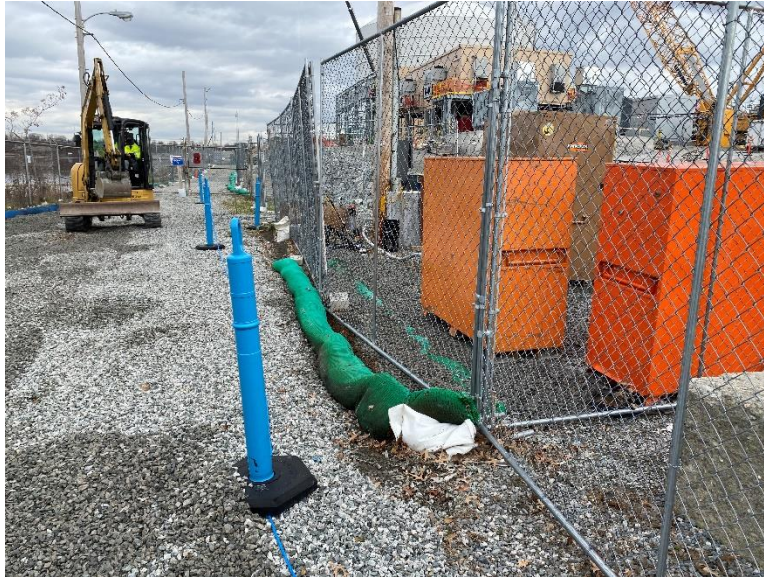
Photo 6: Filtrexx soxx along the south side of the access road to be extended.
